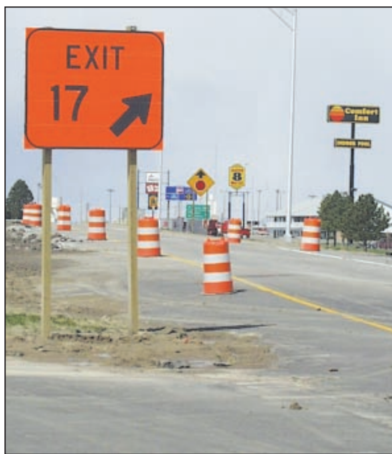
The westbound ramps of the west Goodland interchange with I-70 (Exit 17) will be closed for about a month beginning Monday.
