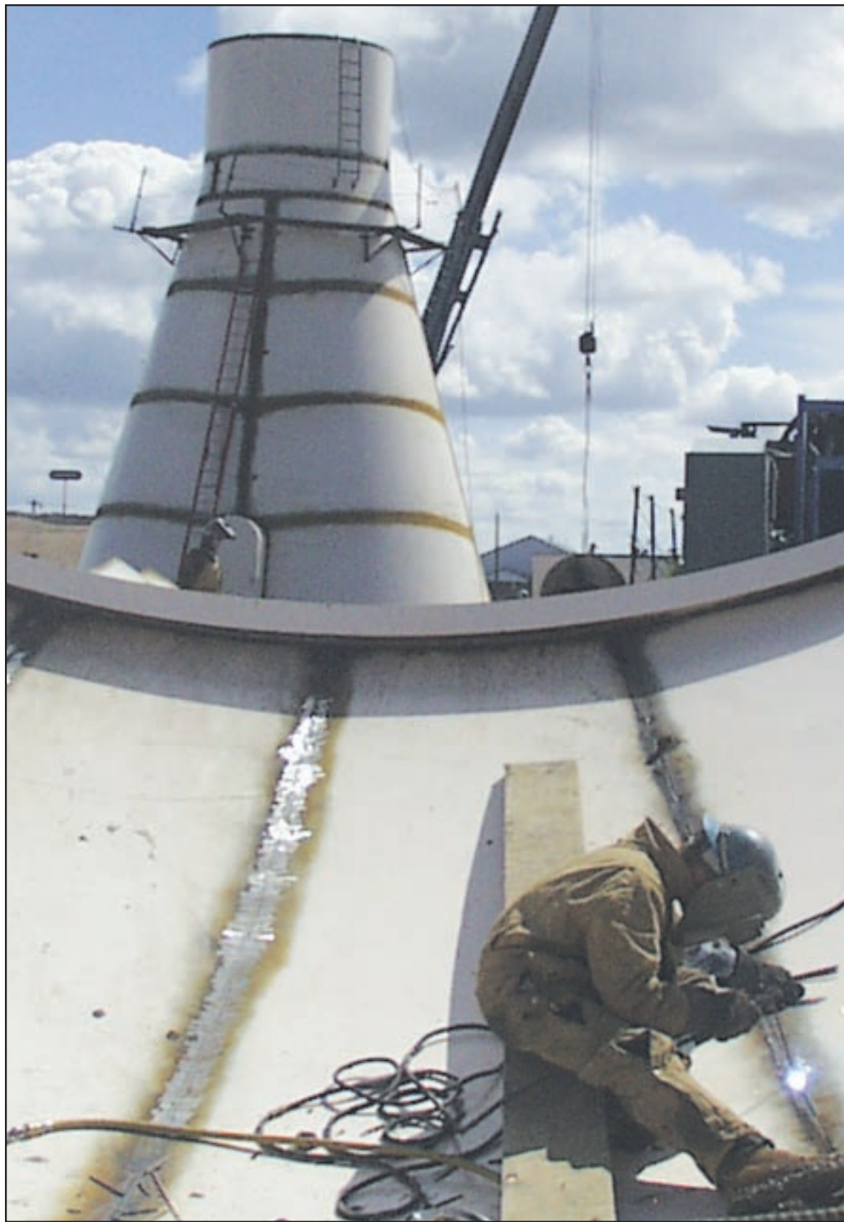
Construction is underway on the Goodland's new 500,000 water tower near Centennial Park in the southwest portion of the city. All the steel has arrived, according to Robert Vasko, project supervisor from Pitt-DeMoine of Pittsburgh, Pa. The first 55-foot section of the tower was up by today, and Vasko said a special 80-ton crane should arrive Friday or Monday, depending on the weather, to handle the erection of the next 55 feet. Mike Berney of Wyoming is already welding on a section of the water ball which will be the top of the tower. The project is expected to take about three months for all the welding, and then a month or two for the painting and finishing.
