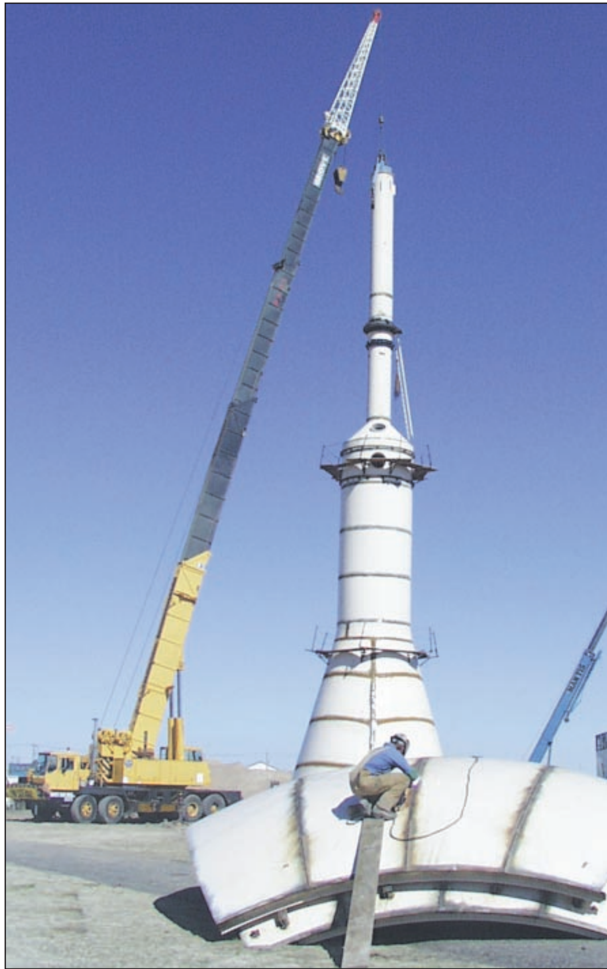
Looking like a launch pad at Cape Kennedy, Goodland's new water tower continued to rise into the air Saturday when the 80-ton crane arrived. Brad Heer, project superintendent, said the good weather allowed the crew to get the interior pipe completed to its 110 foot height. He said an internal crane will be used for the rest of the erection, because the large crane cost $165 per hour. Heer said the welding crew was working on interior joints, and expected to begin the outside work later in the week. Several of the outside sections of the tank itself have been completed, and they will be swung into place beginning the end of the week if the good weather continues. The 500,000-gallon water tank is being built by Pitt-DeMoine of Pittsburgh, Pa.
