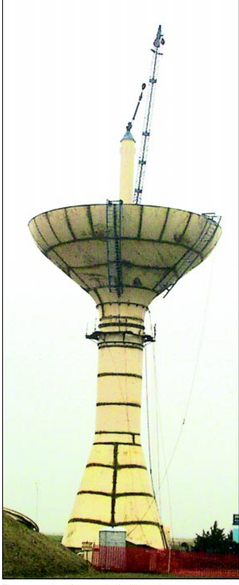
The construction of the new half-million-gallon water tower at the southwest corner of Goodland continues, with the work to be completed by the middle of July. The tower is being built by Pitt-DeMoine of Pittsburgh.
