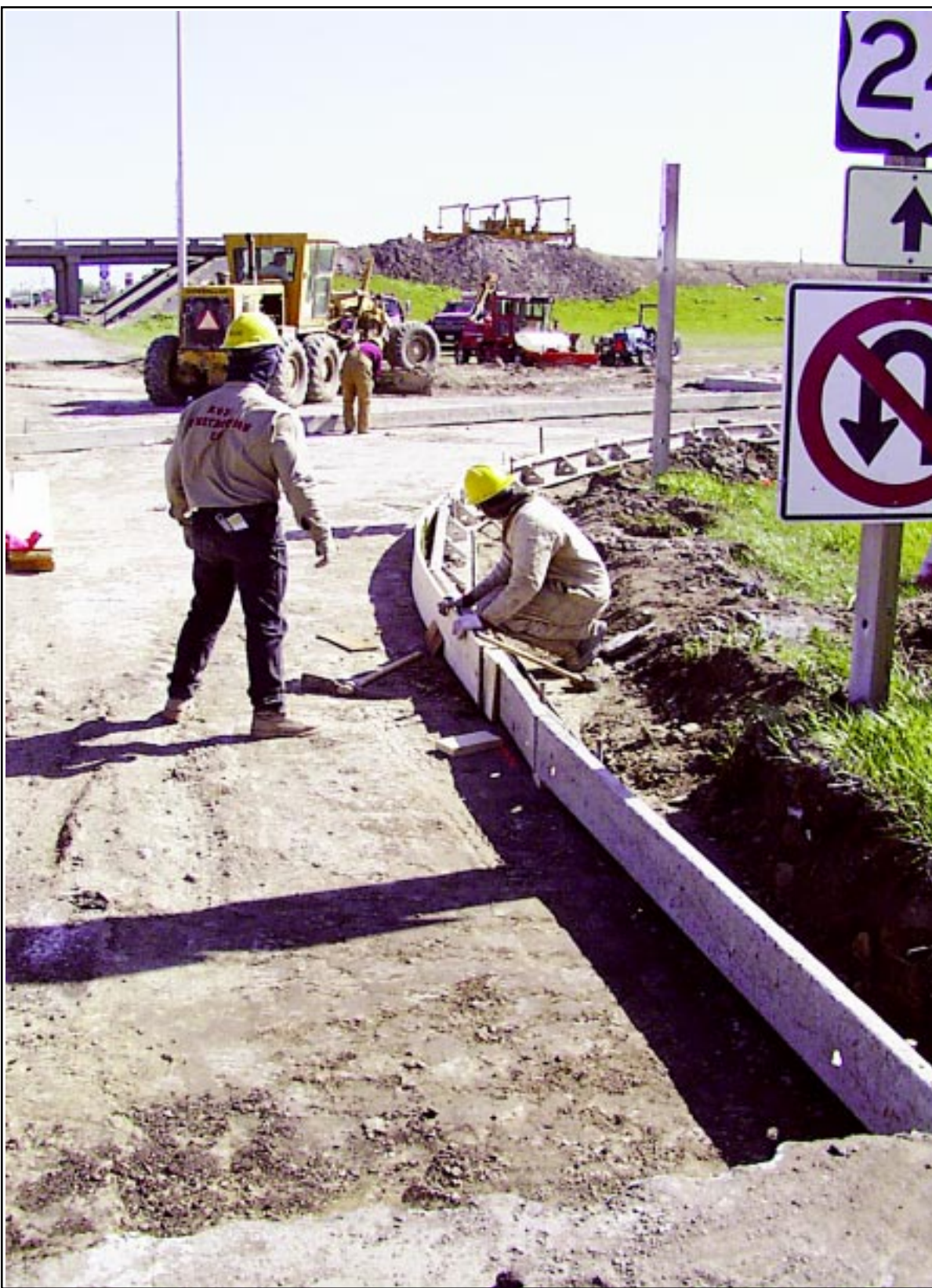
Workers from Koss Construction of Topeka prepared the concrete curb and gutter forms for the west-bound on-ramp of I-70 Thursday afternoon. The west Goodland exit has been poured but is not expected to open until May 21
