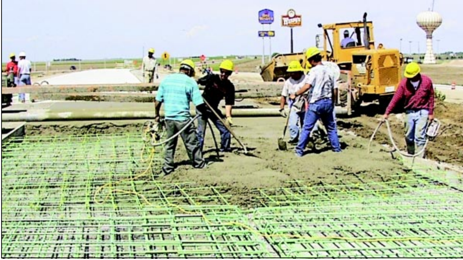
The huge concrete paving machines are working their way eastward between Goodland and Edson laying a new ribbon of highway, but when a bridge is approached the larger machines give way to the more manual
