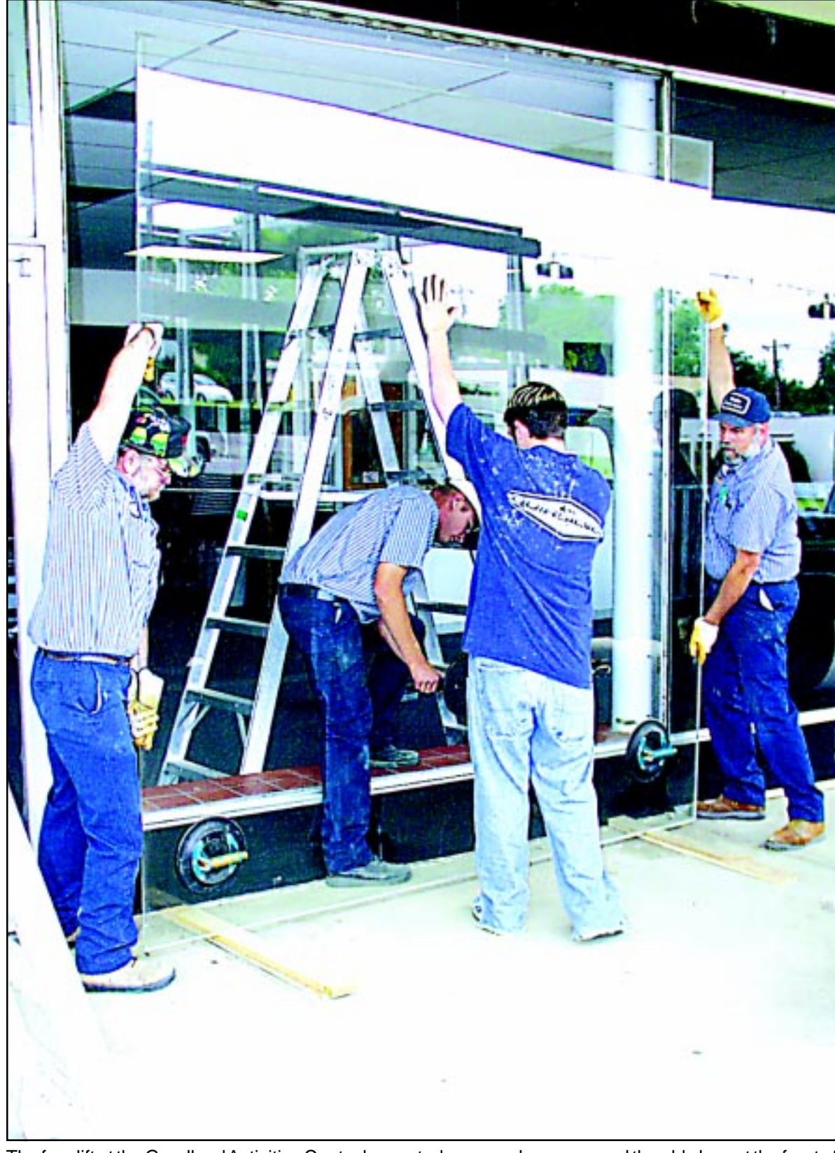
The facelift at the Goodland Activities Center began today as workers removed the old glass at the front of the building. The panes being removed measure 107 inches tall by 101 inches wide and weigh in at over 300 pounds each. Dependable Glass of Goodland is removing the glass. New, energy efficient windows will replace the old. Removing the glass were (left to right) Darrell Rohr, John Studer, Nathan Elliott and Tom Rohr.
