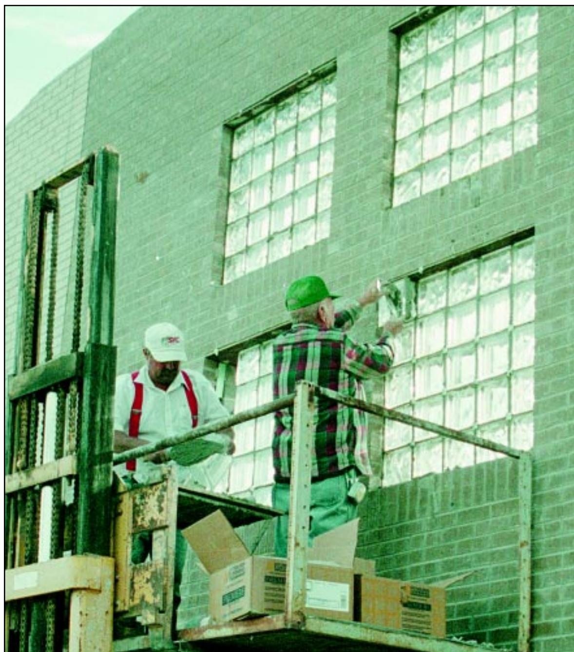
The block work on walls is almost complete at the Max Jones Fieldhouse. The Ginn Brothers are the subcontractors for the masonry. Superintendent Marvin Selby said they have done a good job, and should finish their work sometime next week.
