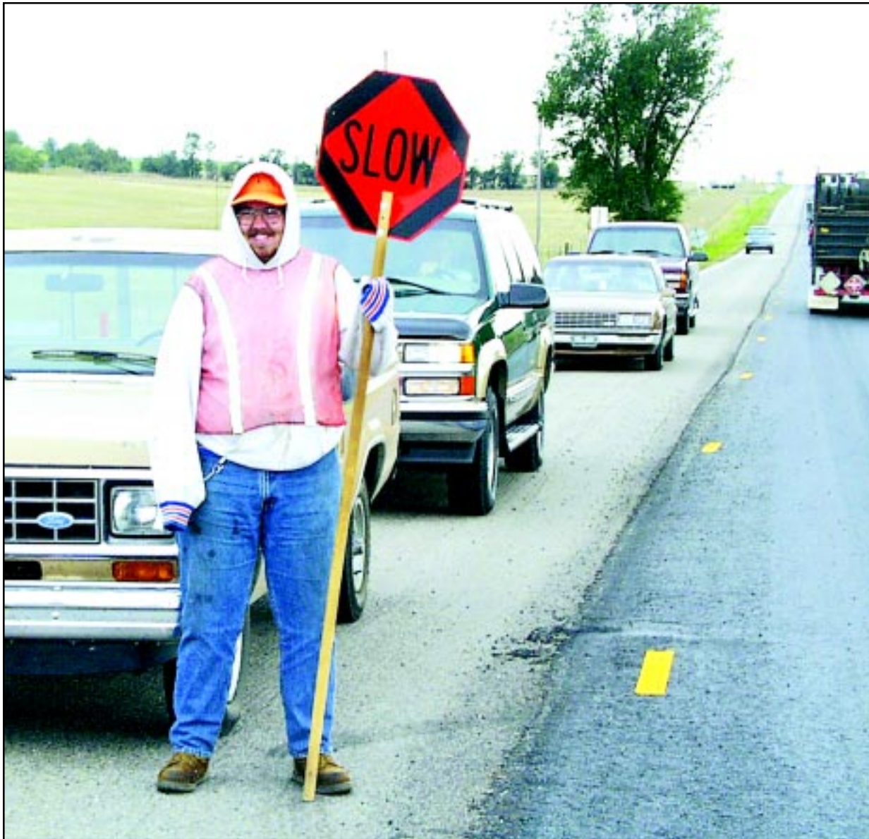
Dustrol has begun resurfacing K-27 north of Goodland, and delays should be expected by travelers. The road will be resurfaced to the county line, and the job should take about two and a half weeks. Photo by Charlie Baker/The Goodland Daily News
