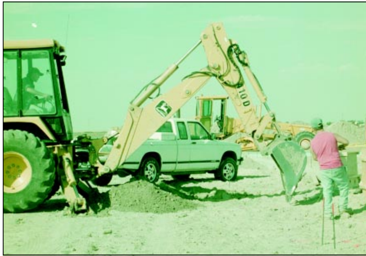
Bill Branch, Castle Rock, Colo., ran the backhoe at the construction site of Wheatridge Acres last week as work began on the assisted-living center. The project is being built by Goodland Assisted Living, L.L.C. Photo by Janet Craft/The Goodland Daily News
