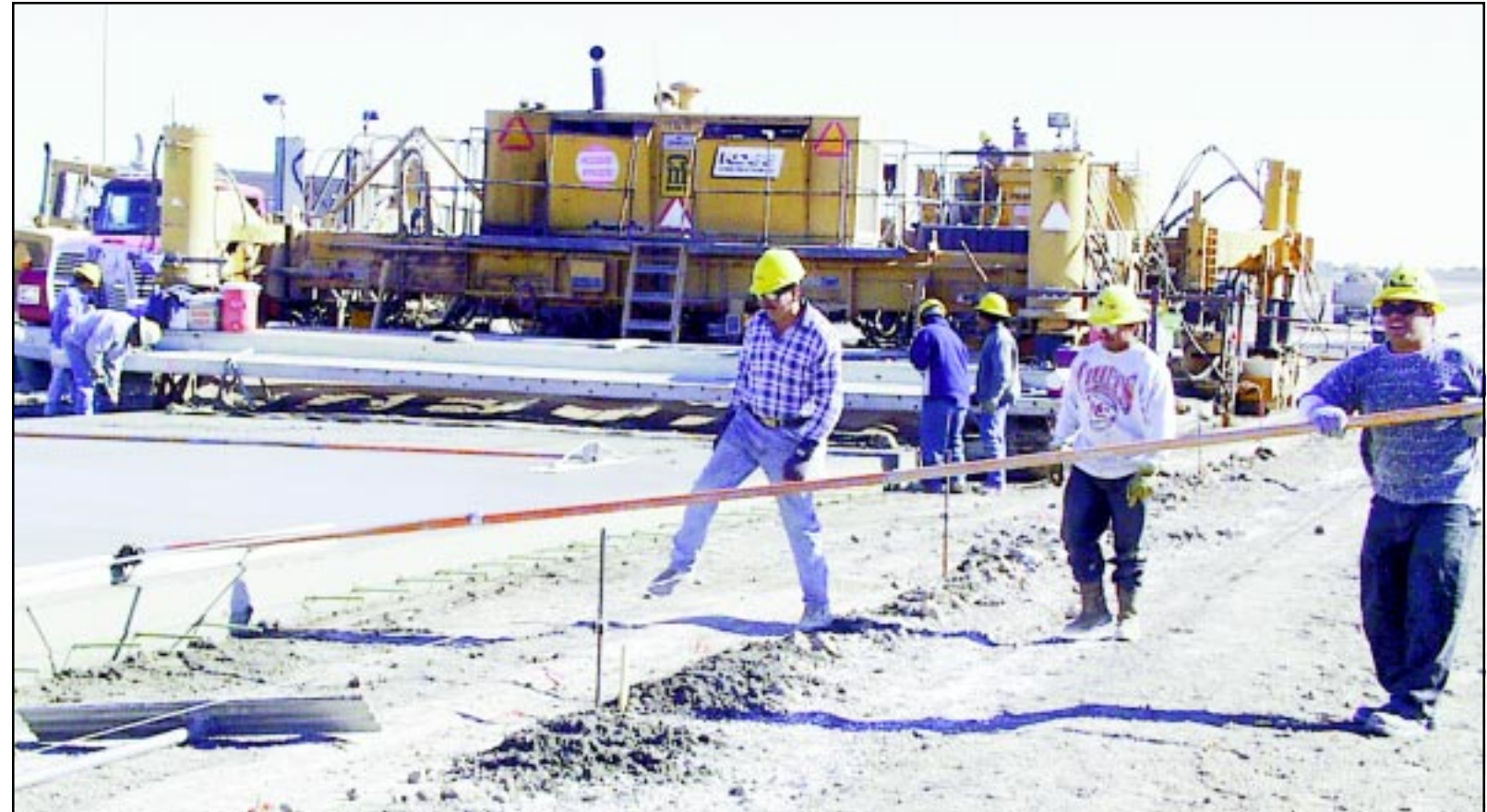
Workers from Koss Construction laid concrete on the eastbound lane of I-70 near the K-27 exit this morning. The big machines can put down about three quarters of a mile a day in good conditions.
