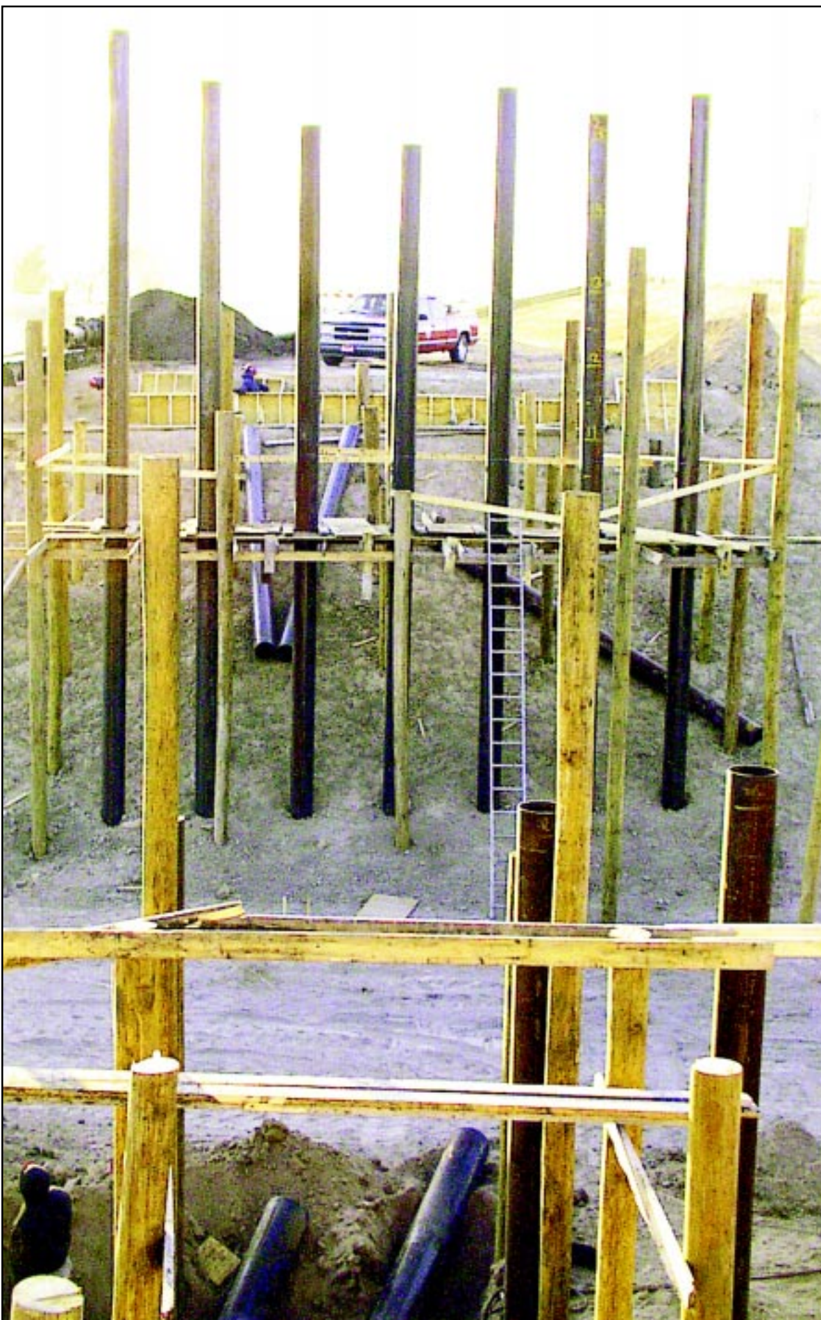
A crew from Reece Construction out of Scandia worked on the replacement bridge west of Goodland on old U.S. 24 on Tuesday. A worker said the good weather has allowed the project to move ahead of schedule, and if it continues, the bridge may be completed sometime in December.
