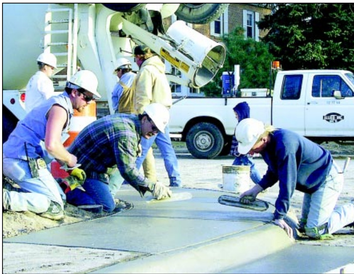
Allen Werth (second from left) and Toby Rupp (right), Allied Inc. workers, smoothed the concrete poured for a portion of a sidewalk at Sixth and Main late Wednesday afternoon. It was part of a bigger job, which replaced bricks in the dip pan of the intersection with concrete.
