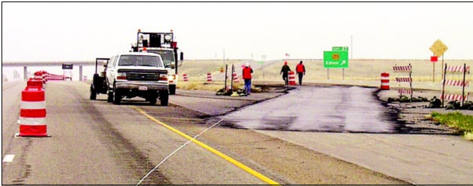
Despite a gloomy beginning to spring this morning, crews from Trancon of Lincoln, Neb., were working near the Edson ramp, preparing to move traffic back onto the eastbound lanes of I-70. Koss Construction is planning to begin work Tuesday. Photo by Tom Betz/The Goodland Daily News
