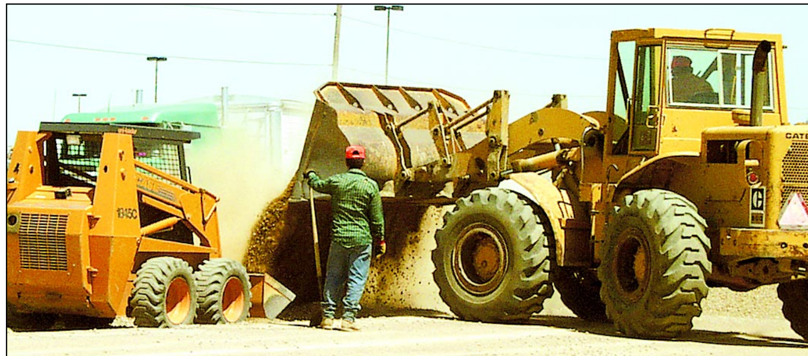
On Tuesday, road workers began filling in the holes that they had dug in the median on K-27, which will be paved over during the summer's construction project. Today, they planned to start milling the south part of the
