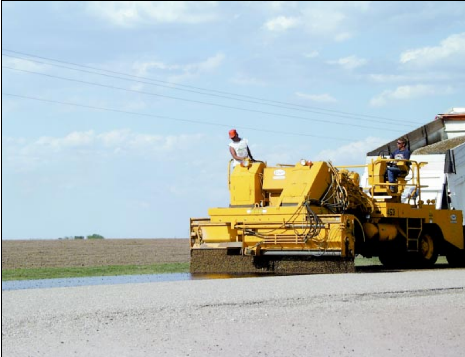
Chip sealing work started Wednesday on the west bound lane of K-24 between Goodland and Kanorado. Traffic is reduced to one lane for a
