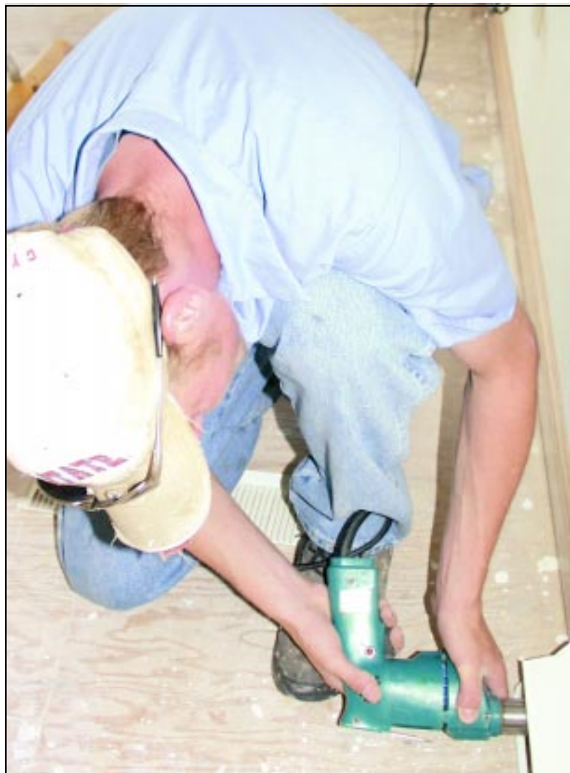
Carpentry student Ryan Bowman installed vents over registers Thursday morning in a house Northwest Kansas Technical Students built this year. It will open to the public on Sunday.
