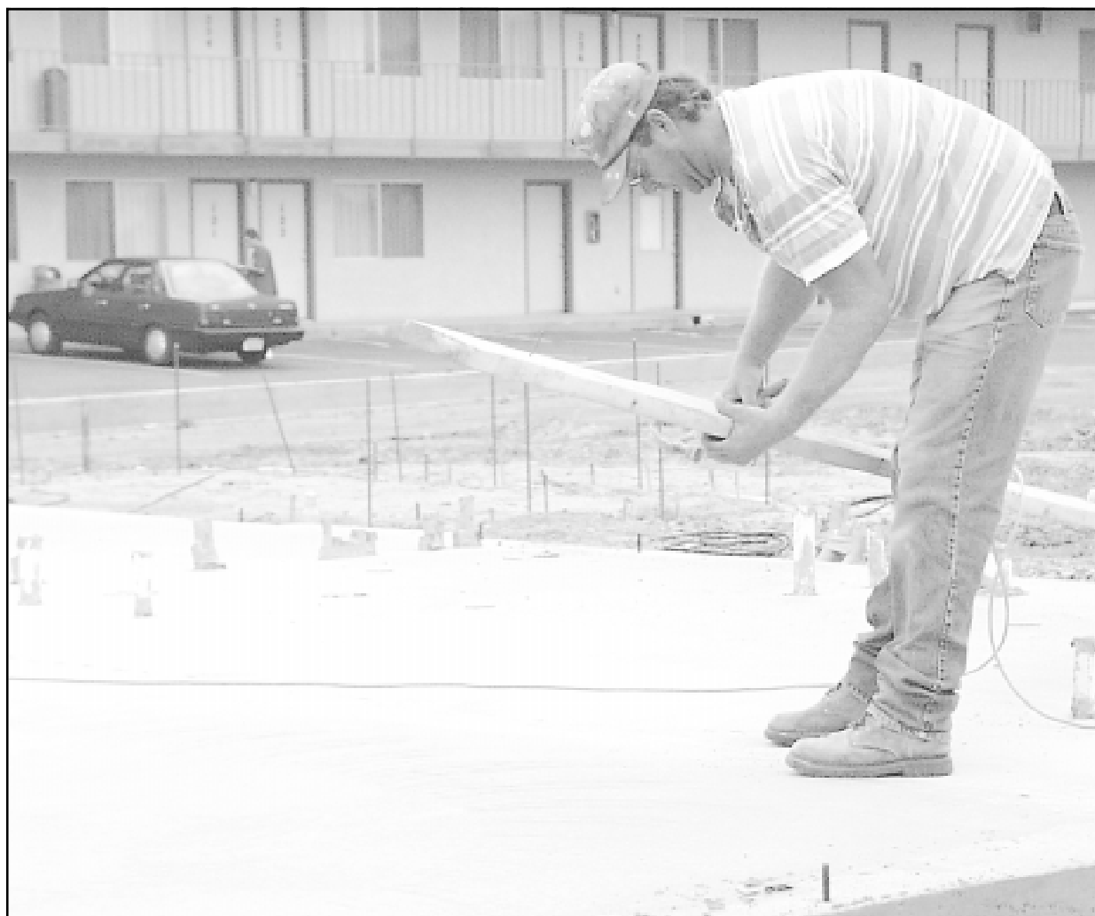
Curt Sawatzky with Kruse Construction of Goodland removed nails from a piece of lumber which had been part of the form for the concrete slab poured at the new Dairy Queen store along K-27.
