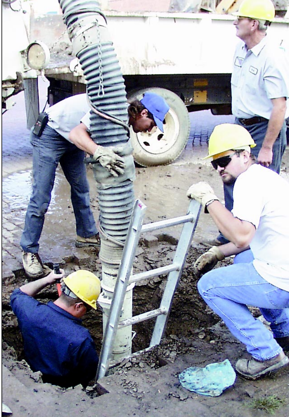
City crews sucked mud and dirt out of a hole in front of the Sherman Theatre on Main Street today as they worked to locate a leaking water line. Randall Stasser, in the hole, directed the nozzle as Neal Thornburg assisted from above. Travis Gillihan held the ladder while Dean Townsend supervised. Once the line was found, the crew pumped water out to enable them to repair the leak. Photo by Tom Betz / The Goodland Daily News
