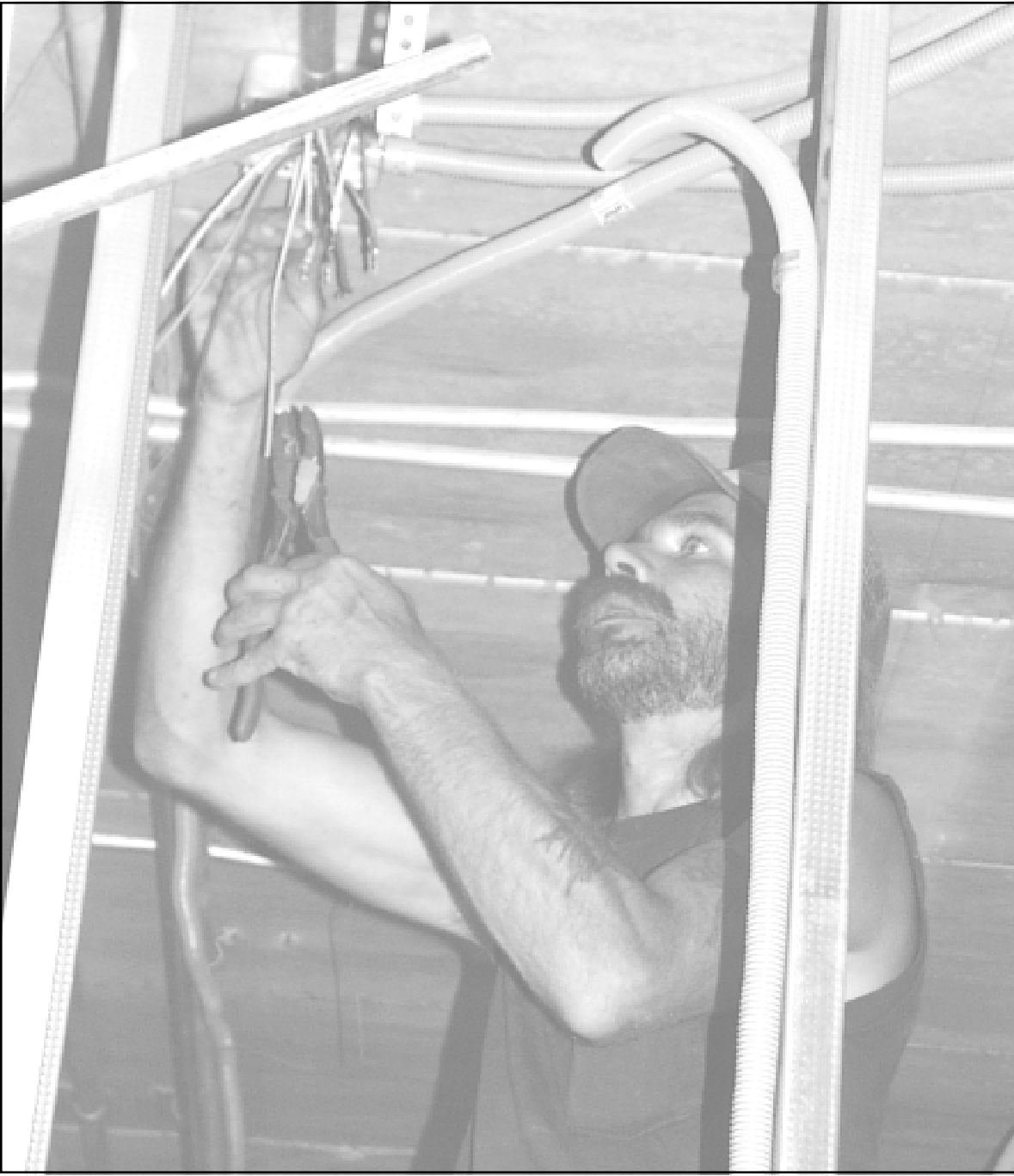
Rhoads Construction of Goodland is remodeling the inside of the old Medical Arts Clinic at 520 Main for offices. Tony Pennington, who works for Marty Electric in Goodland, twisted electrical wires Wednesday afternoon in one of the rooms.
