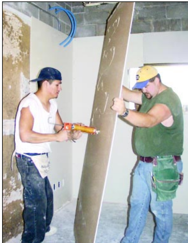
Carpenters worked Friday morning on remodeling the old Medical Arts Clinic. Paul Medrano (left) applied adhesive to a piece of sheet rock, while Will Weisshaar held it. Photo by Janet Craft/The Goodland Daily News
