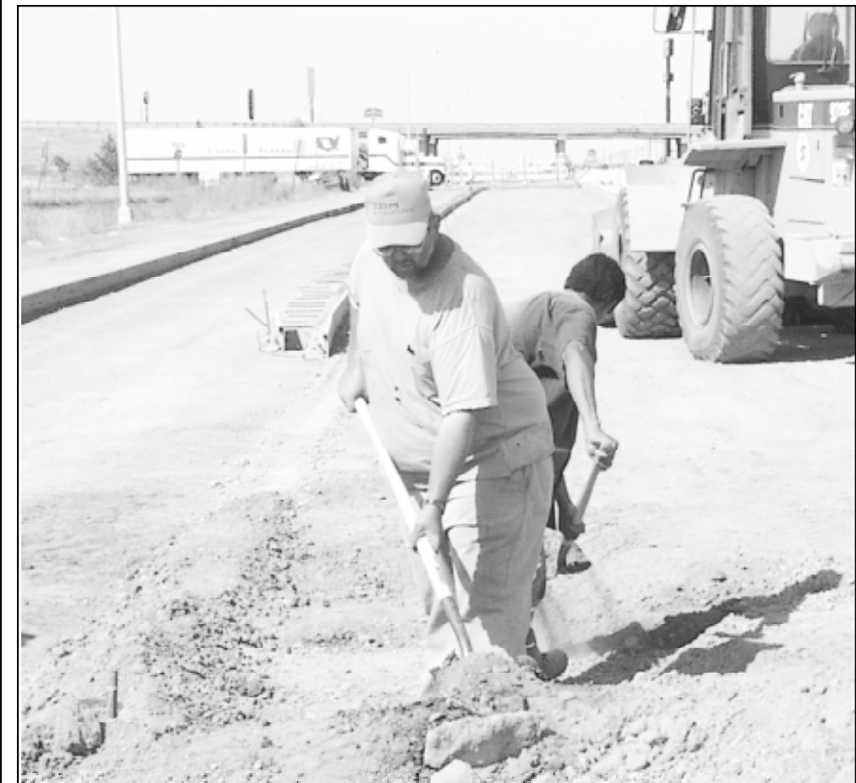
Workers with Smith Sand and Gravel of Garden City were preparing the base on K-27 before concrete is poured. Dan Hershberger of Goodland (front) and Luis Ortiz of Garden City shoveled dirt Monday afternoon near the entrance of the Total Petroleum service station south of I-70. Photo by Janet Craft/The Goodland Daily News
