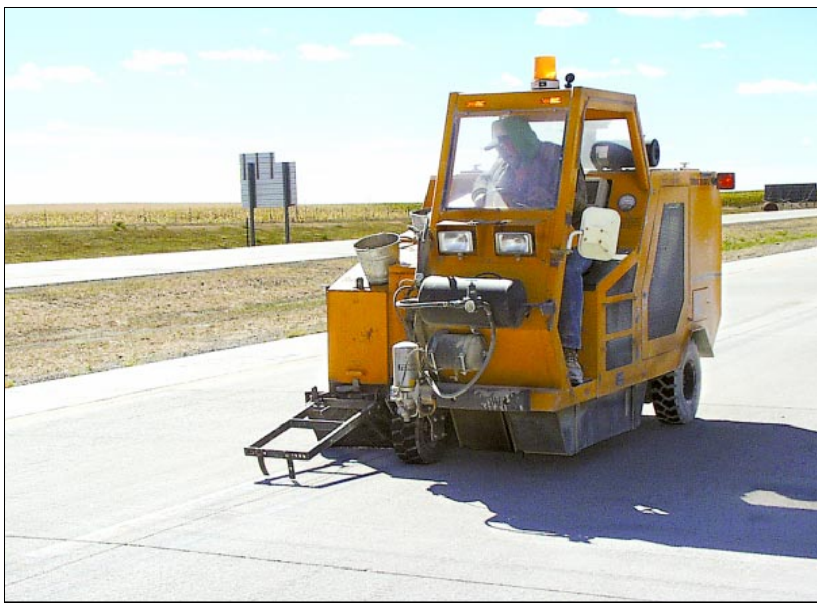
Gary Trafcon (above), owner of Trafcon, a construction firm in Lincoln, Neb., used a machine to scrape temporary stripes from the westbound lanes of I-70 near Edson Wednesday afternoon. The firm is finishing the last phase of the I-70 rebuilding project that started a year and a half ago. Ernest Knight (below) used a power washer to blast away the striping tape. Photos by Rachel Miscall/The Goodland Daily News
