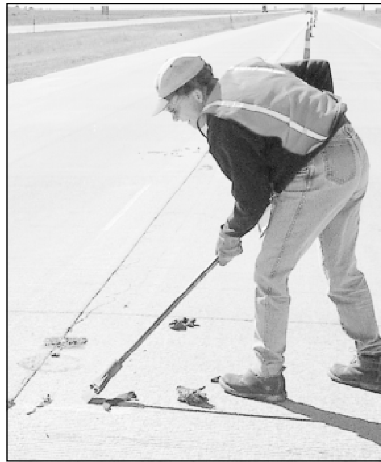
Pat Colsom, with Trafcon, a construction firm from Lincoln, Neb., scraped tar off the westbound lanes of I-70 near Edson Wednesday afternoon. The tar once held tubes and reflectors in place while another company repaved the highway with concrete. Trafcon is removing barriers and temporary paint as the final stage of the repaving project. Photo by Rachel Miscall/The Goodland Daily News
