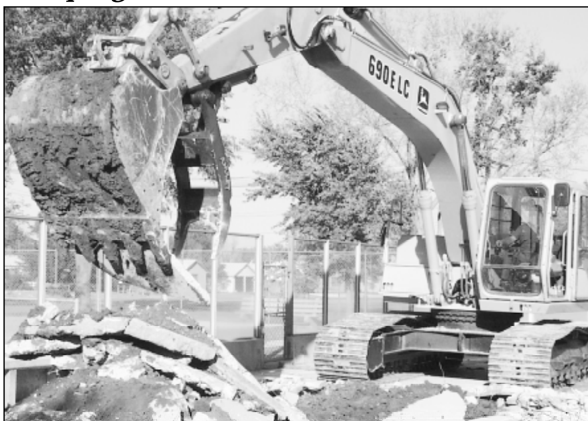
Wilbur Tiede of Tiede Construction was tearing up the cement at the old Goodland swimming pool in Steever Park on Thursday afternoon. The pool leaked and has been closed since last year. It is being replaced by a new water park nearby.
