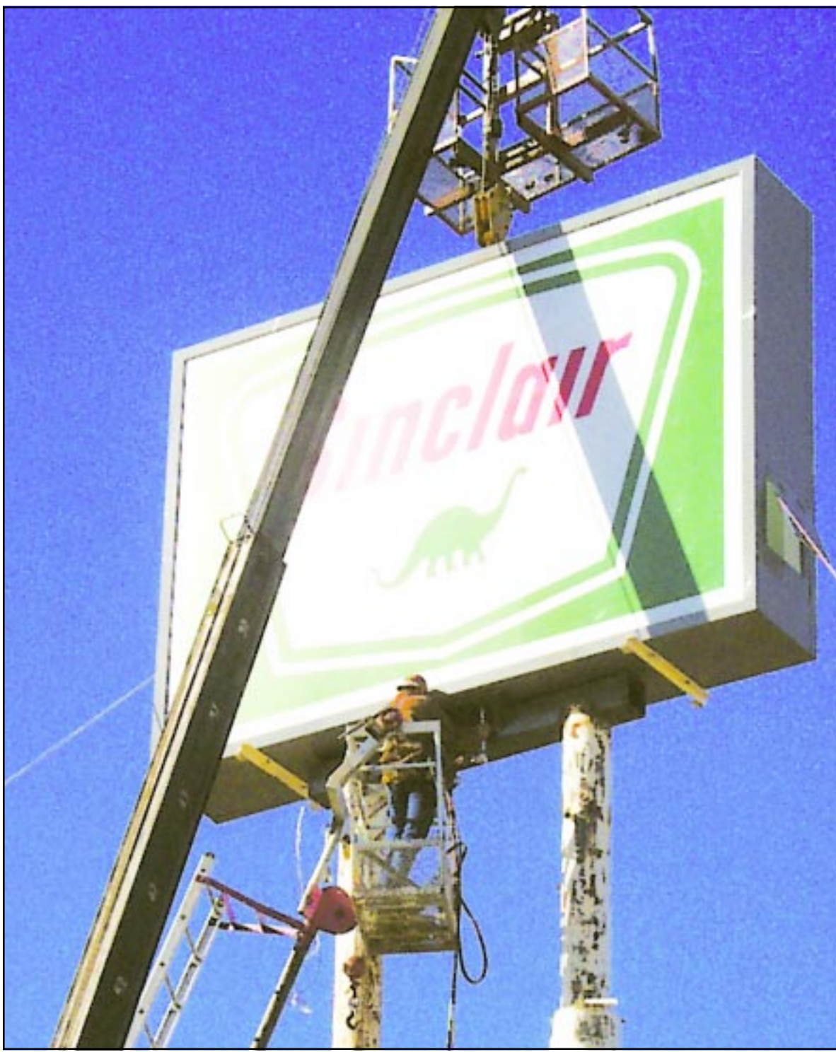
Workers put up a new Sinclair gas station sign on Friday. New owners, Pete and Danny Whalen, purchased the old gas station next to Howard Johnsons on K-27, and have been remodeling it for the past week. Photo by Dana Sulsberger/The Goodland Daily News
