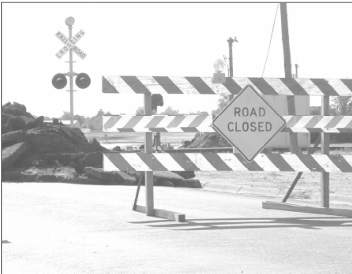
Cherry Street (pictured above), where it crosses the railroad tracks, remained blocked this morning as the railroad crossing, formerly made of wooden planks, is replaced with new concrete panels. The crossing is to be closed until this evening. Photo by Dana Sulsberger/The Goodland Daily News
