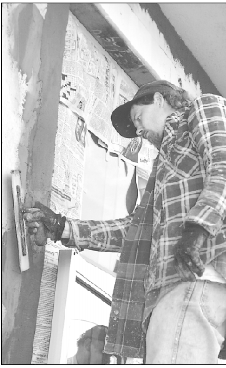
Steve Goalden of Linden Construction in Colby spread a layer of stucco Monday afternoon on the outside of the Goodland Activities Center. The work is being done as part of the remodeling that has been going on at the center. An open house will be held from 5:30 to 7 p.m. Friday to view the renovations.
