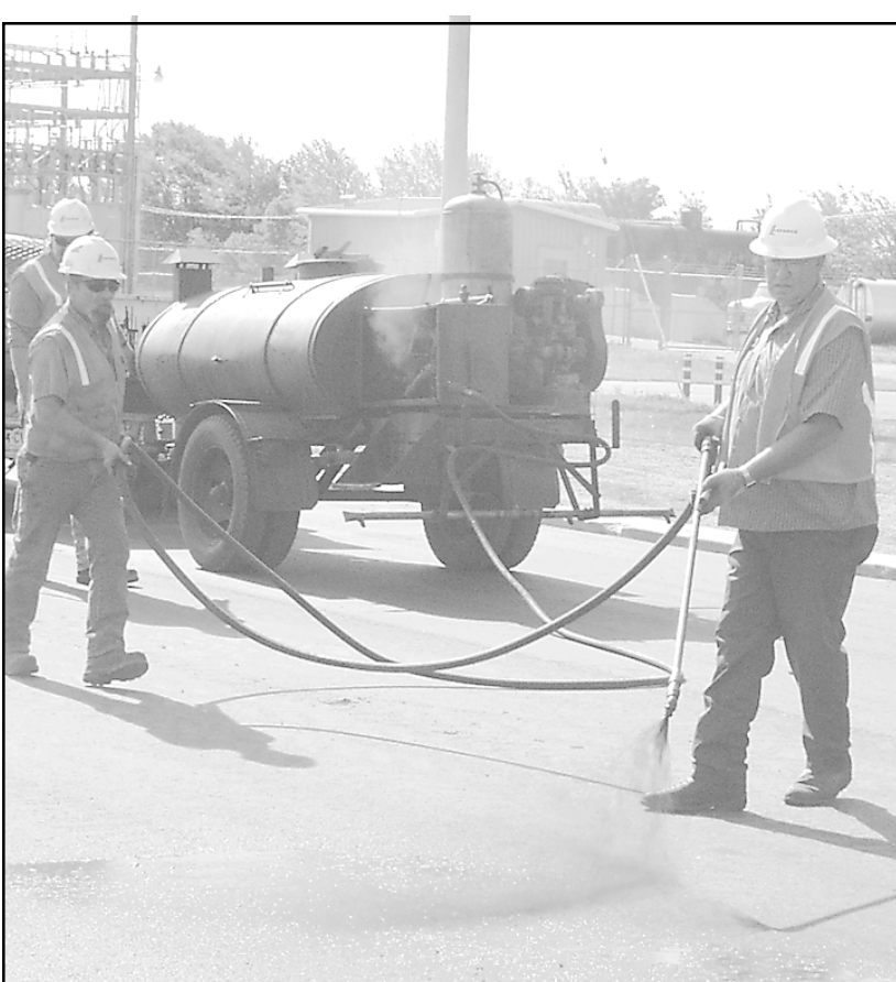
Jerry Andrews with Lafarge, an asphalt paving company from Burlington, sprayed oil this morning on the first layer of asphalt on the access road to help bond it with a second layer.
