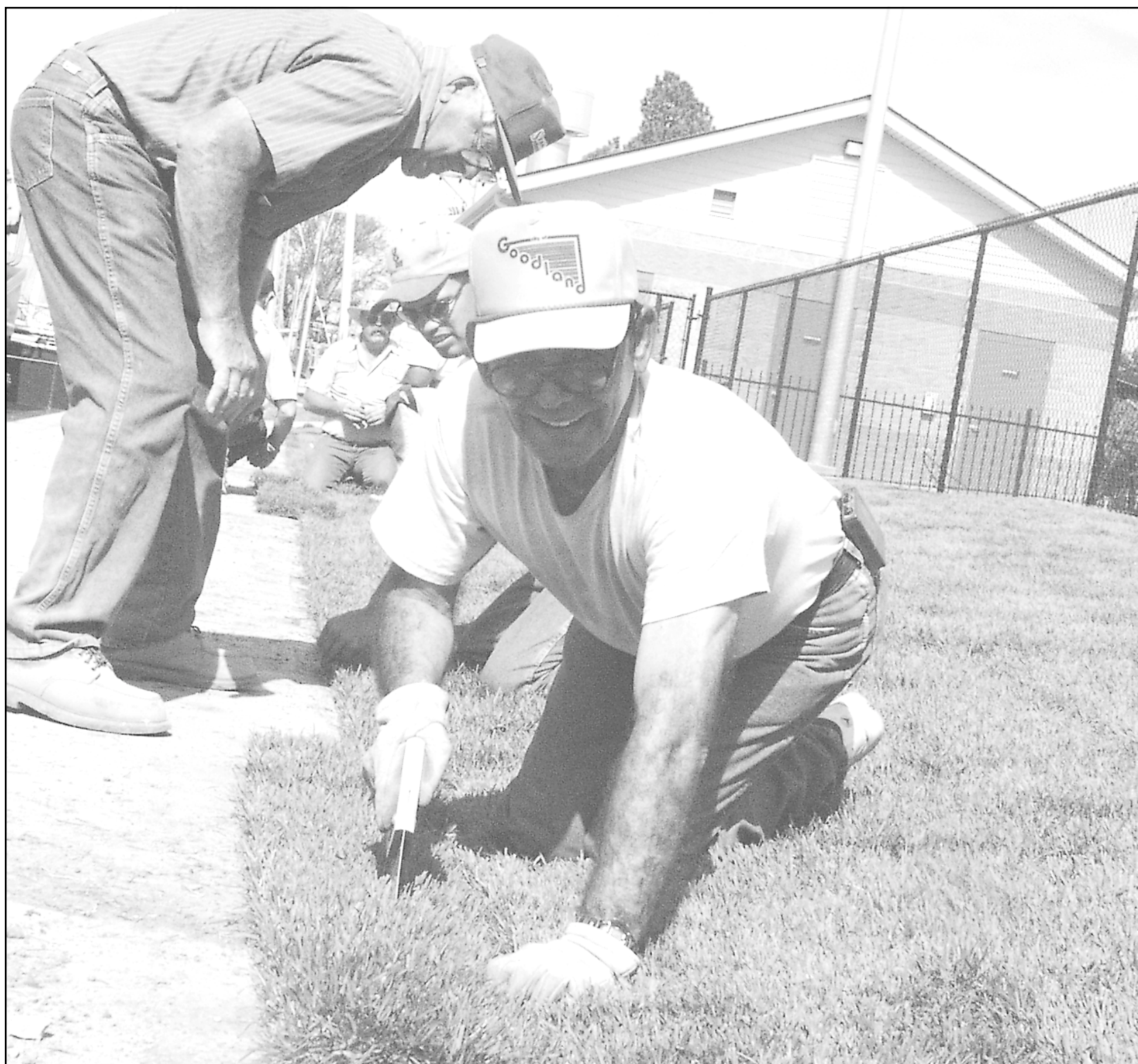
City employees began laying sod this morning at the new Steever Water Park in Goodland. Manuel Hernandez cut sod even with the edge of the sidewalk as other crewmen inspected his work. Photos by Janet Craft/The Goodland Daily News
