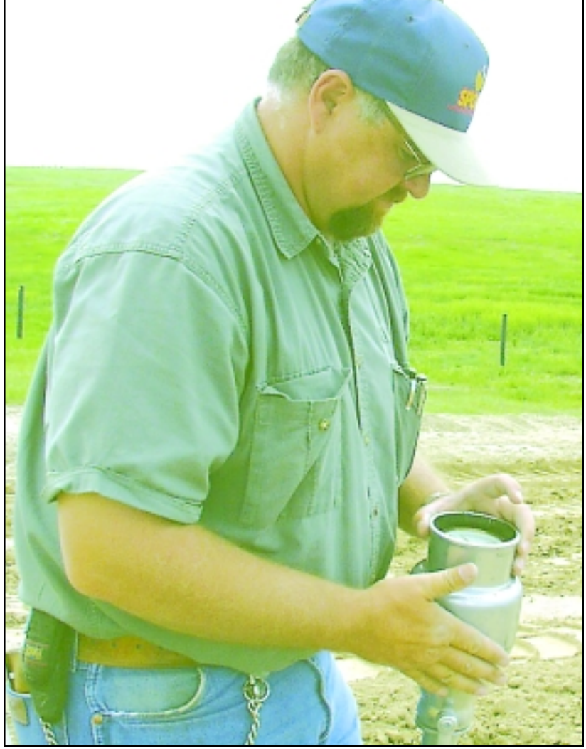
Randy Most, engineering technician for Kansas Department of Transportation, tested the compaction and moisture of the K-27 roadbed to make sure it meets specifications. Photo by Tom Betz / The Goodland Daily News
