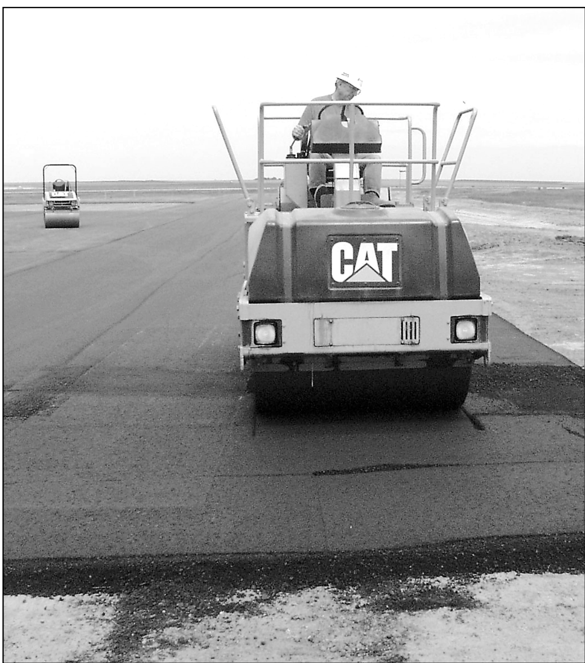
A worker from Lafarge Corp. rolled the first three inches of pavement Thursday south of the new hangars at Renner Field. The project is part of an upgrade which includes two new private hangars and a new taxiway out to the crosswind runway.
