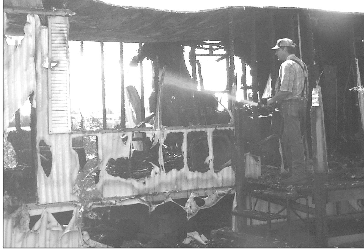
A fireman sprayed water into the living room of the trailer where a mother and two of her three children were killed when fire engulfed their home early Monday morning in southwest Goodland.
