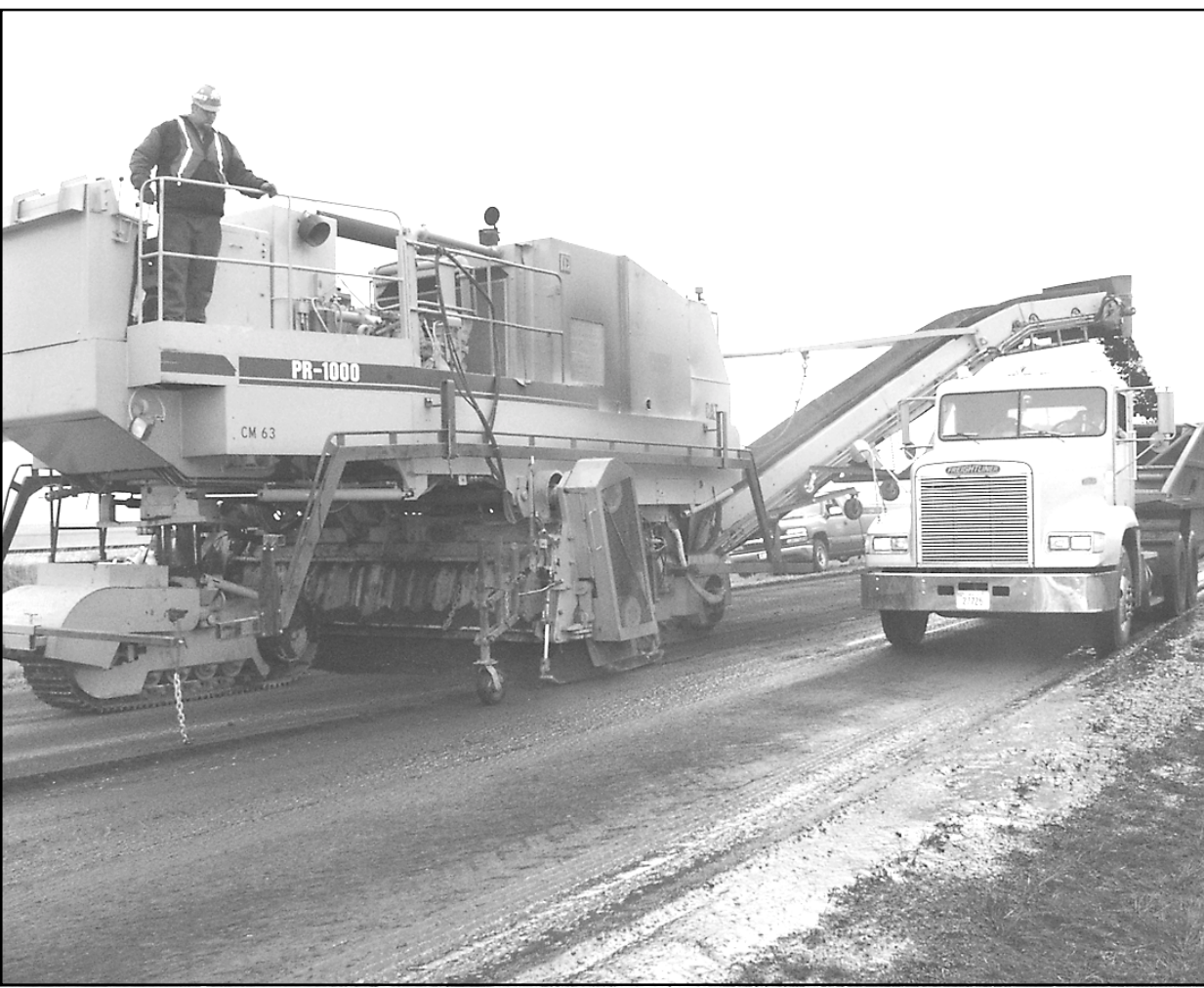
Workers for Düstrol, a construction company from Towanda, milled three inches off a section of Old U.S. 24 east of Goodland Wednesday, while county trucks hauled the material to a site in Edson. The company did the same to a portion of the highway in Goodland on Tuesday. Another crew, from Burlington, will lay new asphalt on both sections. Photo by Rachel Miscall/The Goodland Daily News
