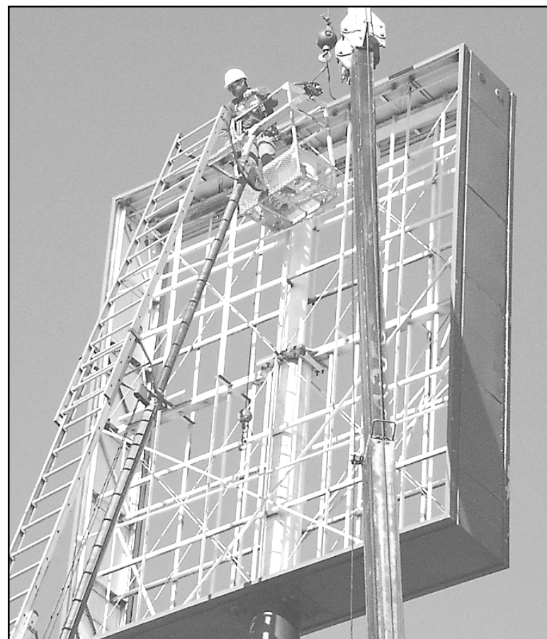
Gary Salzbury, from Commercial Sign Co. of Colby, was installing a new sign for the Economy 9 Motel on K-27 in Goodland. The establishment had been known as Motel 6.
