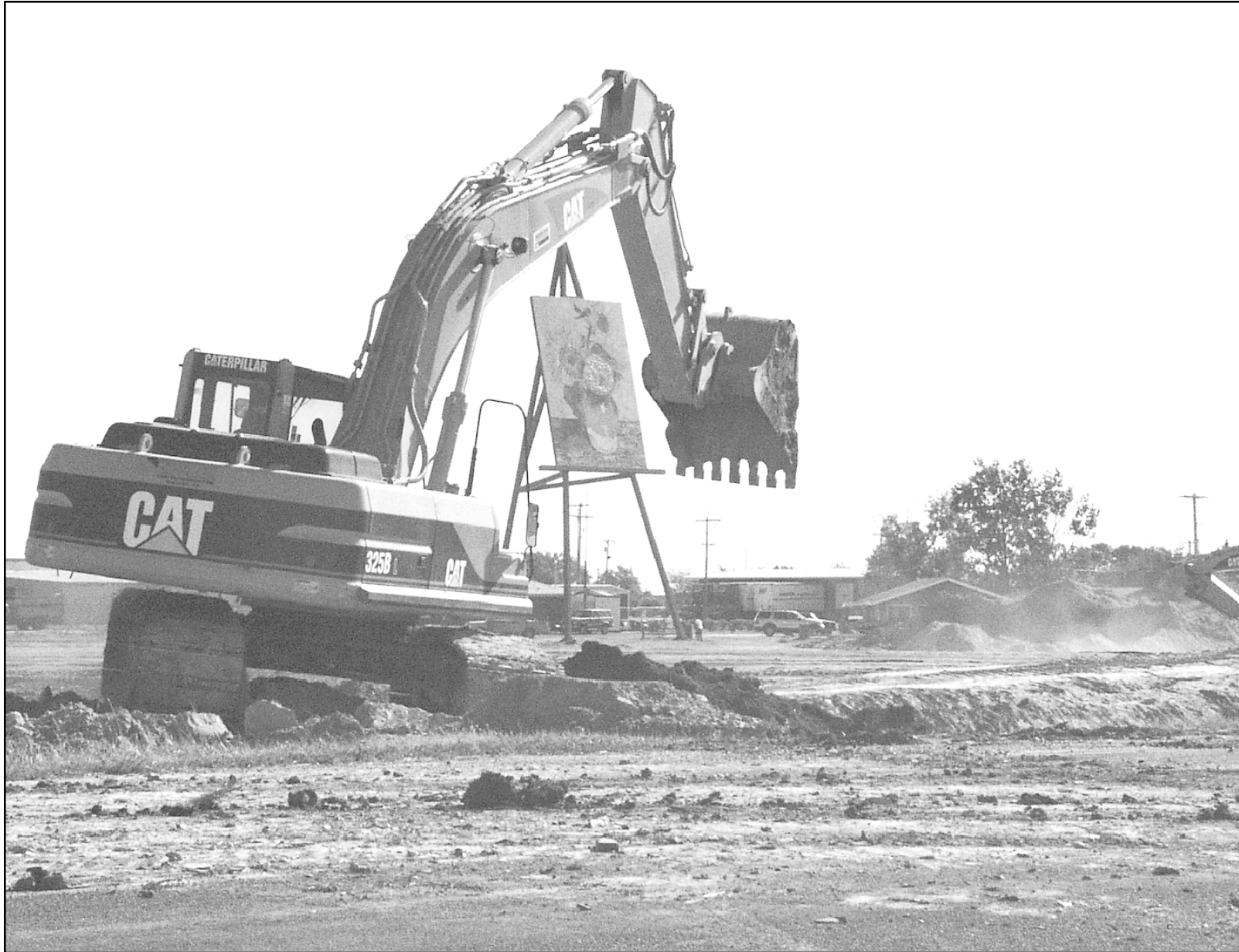
Workers cleared dirt on Friday while working on the Cherry Street project north of Business U.S. 24. The job, which will create a new road and entrance to Goodland, is expected to be completed in October. Photos by Lester Bolen/The Goodland Daily News
