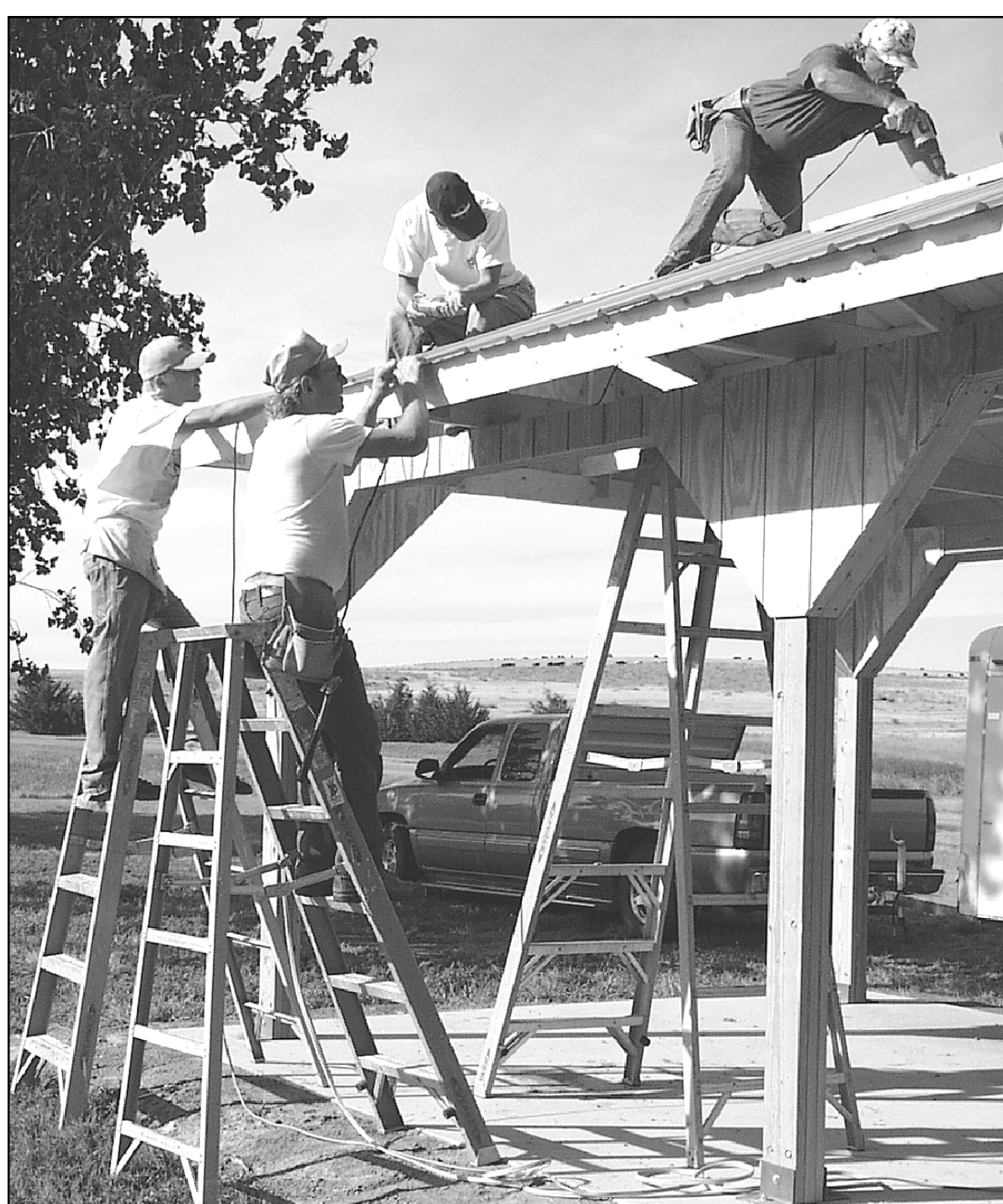
Blake Saint, Bob Evans, Max Saint and Dennis Saint worked on the roof of the new picnic shelter being built at Smoky Gardens on Thursday. The project is being led by Max Saint, who is building the shelter as part of his Eagle Scout Project.
