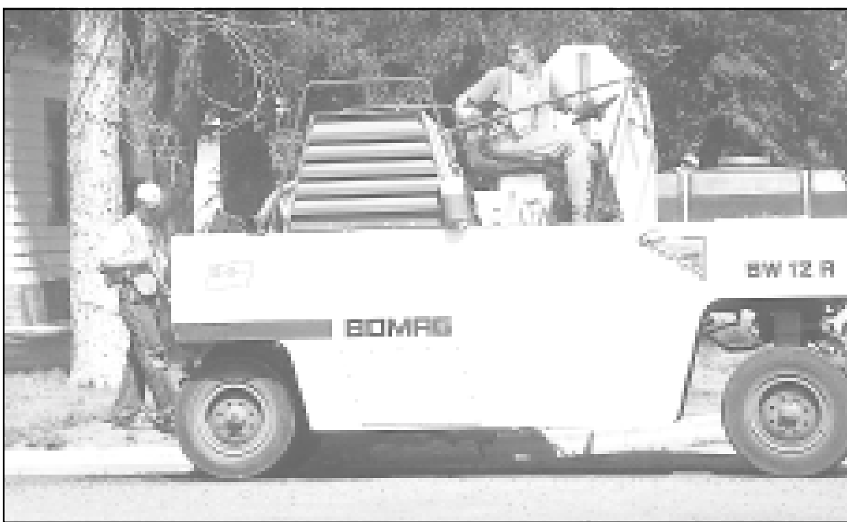
City workers filled in soft spots on Caldwell Avenue on Thursday. The repair work is being done before the contractor begins chip sealing the streets. Photo by Lester Bolen/The Goodland Daily News
