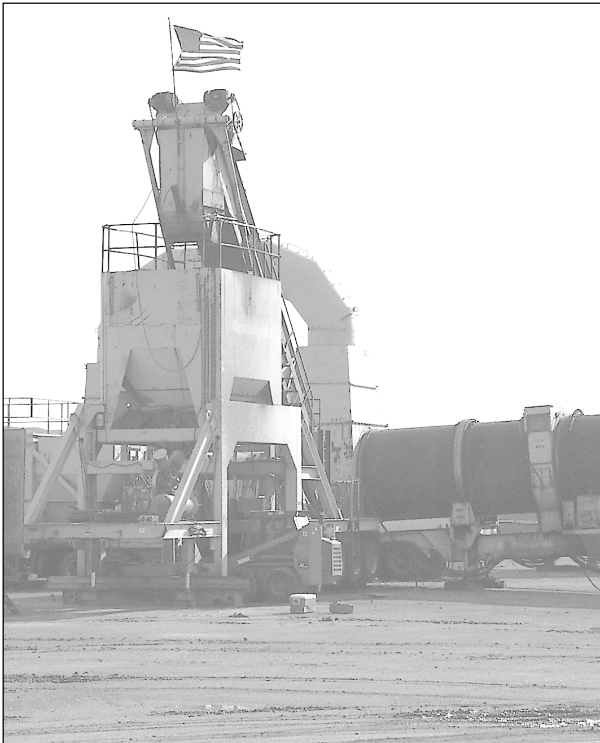
An asphalt paving plant has been erected south of Goodland on K-27, which means that the paving of the road projects around the county should begin on schedule. Photo by Lester Bolen/The Goodland Daily News
