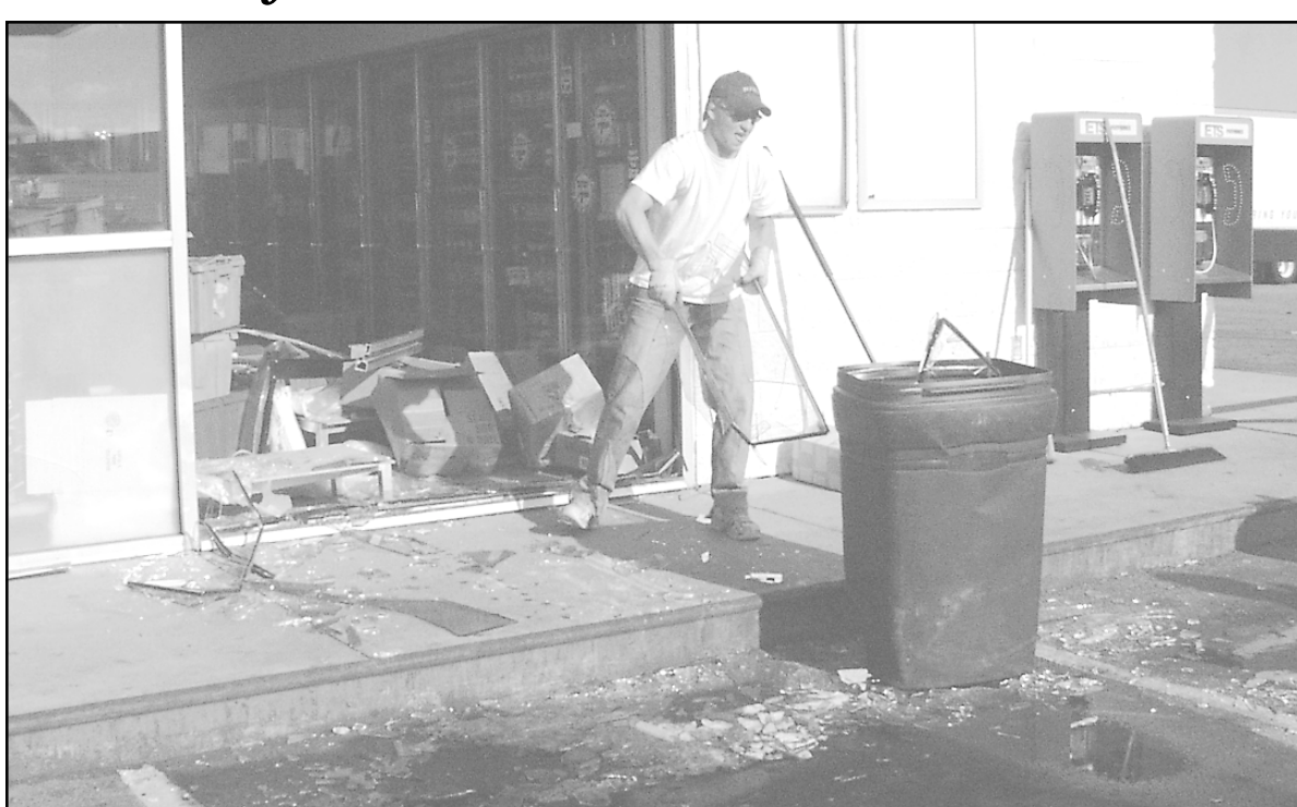
Workers cleaned up at the Total/A & W store on K-27 this morning after a 1991 4-door Mercury, owned by Jesse Sandoval, crashed through the north window around 7 a.m.. J.R. Johnson, a Goodland police officer on the scene, said apparently the car jumped into gear while the driver was inside paying. Police would not release the identity of the driver, as they said the incident is still under investigation. Photo by Reaghan Smith/The Goodland Daily News
