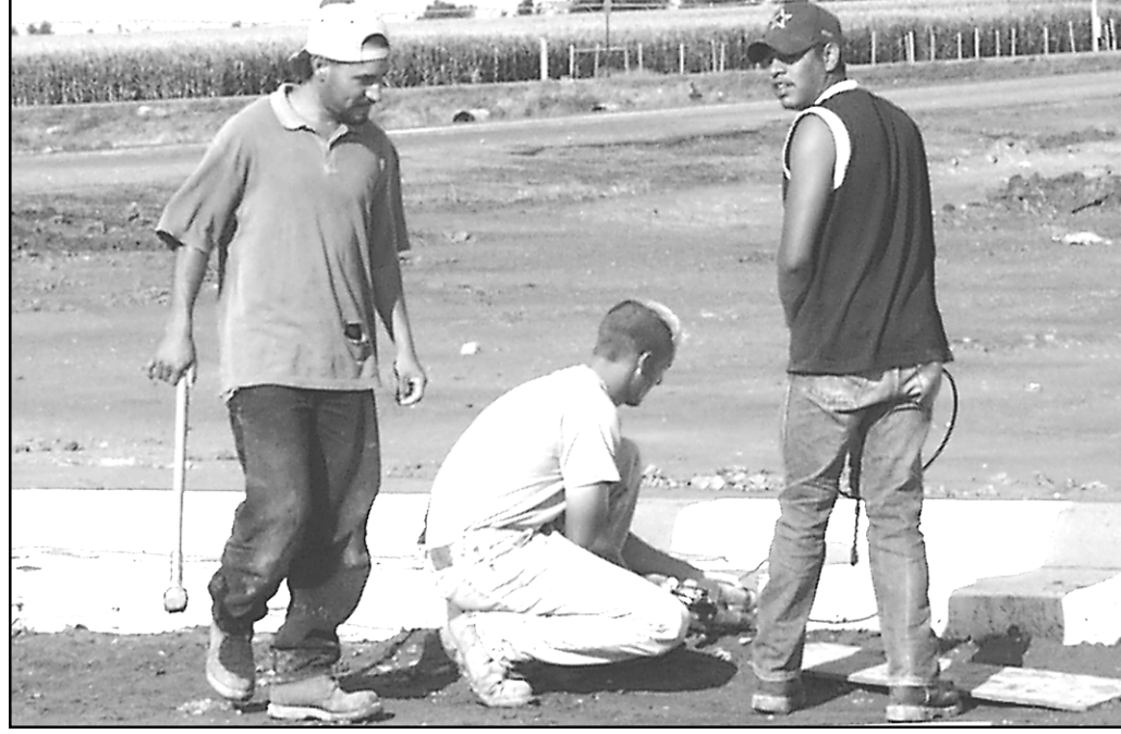
Workers on Wednesday morning smoothed the curb and gutters on a new section of Cherry Ave. at the junction of Business U.S. 24. Ritchie Paving will pave the new road. The old section is closed and businesses along the street are upset.
