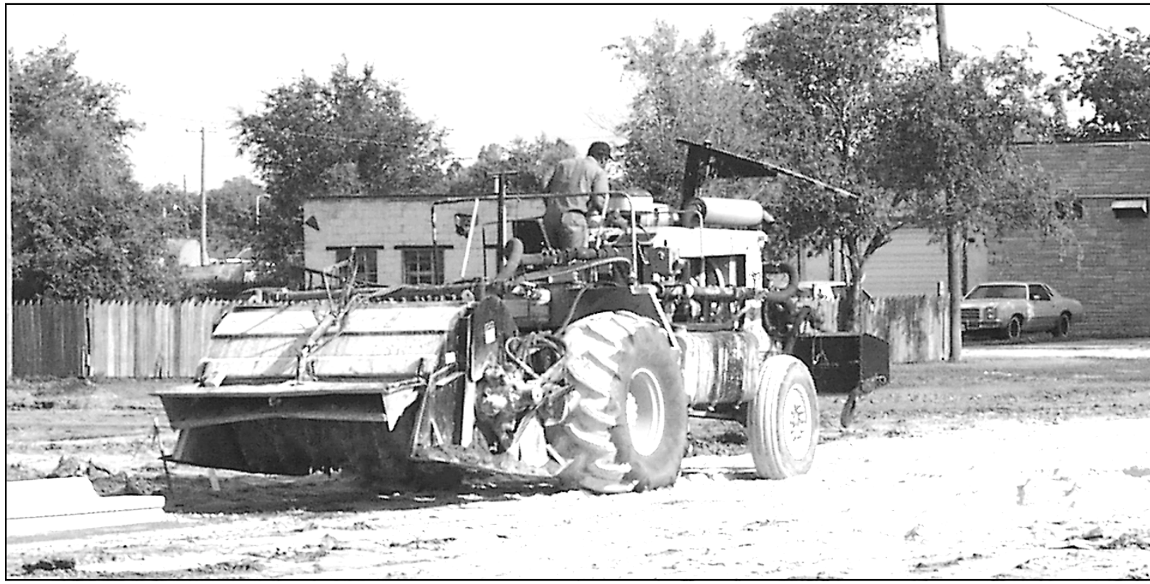
A construction worker smoothed the fly ash that was laid for the base of Cherry Ave. Wednesday morning. Ritchie Paving, a construction company from Wichita, will pave the new road soon.
