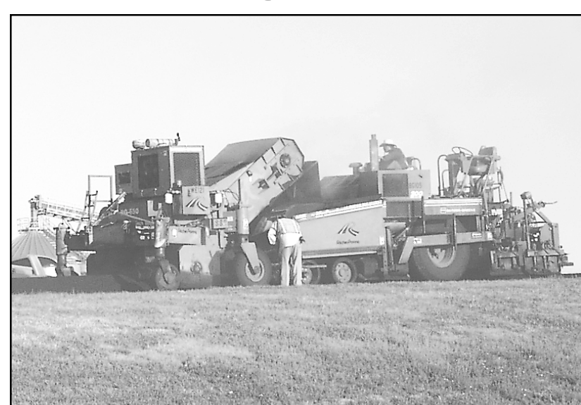
Workers for Ritchie Paving were laying down a layer of asphalt on a section of north K-27 Monday for about a mile north of U.S. 24.
