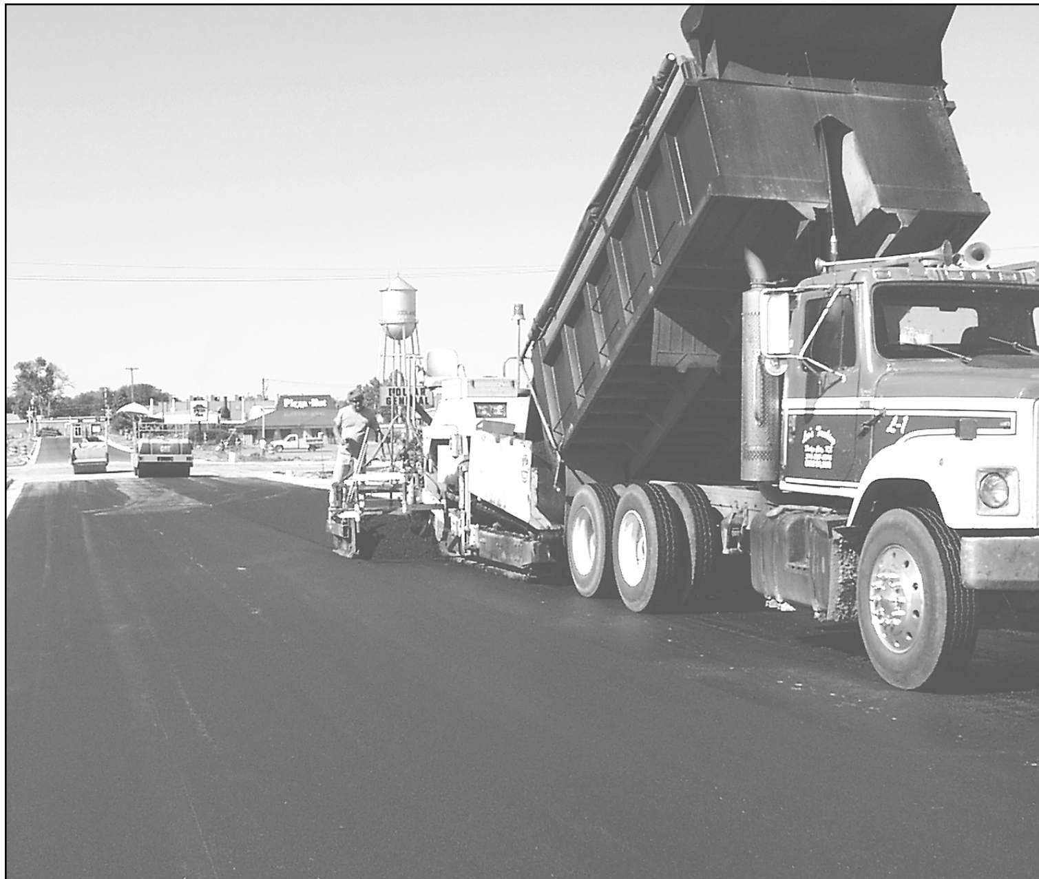
The new Cherry Avenue should be open to traffic on Thursday. on Wednesday, which will allow the road to be opened to traffic. Workers on the paving crew Monday said striping would be done. Photos by Tom Betz / The Goodland Daily News
