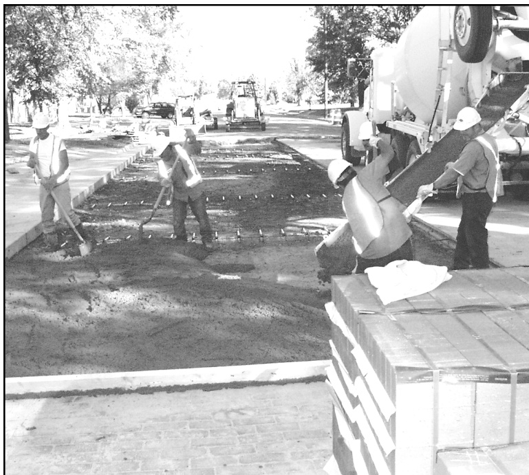
The bricks have arrived for the new intersection at Sixth and Main, and workers from APAC of Hays, were pouring the final sections of the six-inch concrete base Wednesday. Weather had delayed the project. Photo by Tom Betz / The Goodland Daily News
