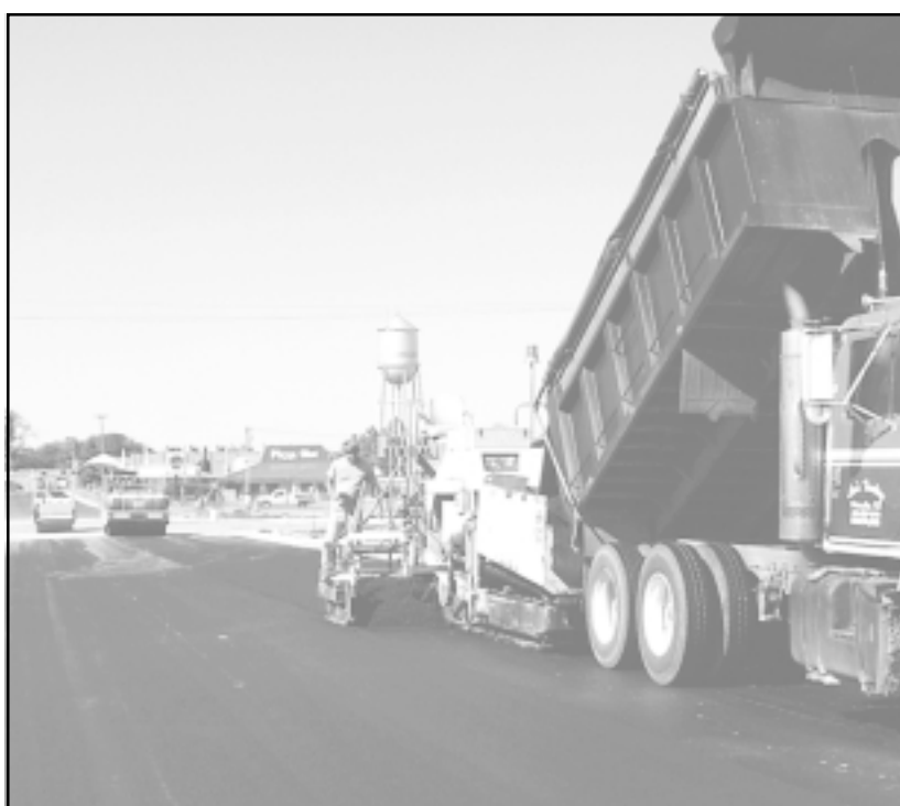
Pavers worked to finish a new section of Cherry Street in August. The street forms a new entrance to Goodland, flanked by a giant sunflower painting and, soon, a new Pioneer Park.
