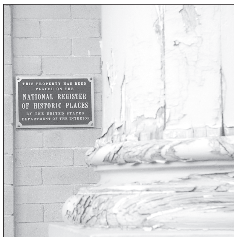
The bases of the columns at the Carnegie Art Center are crumbling and plaster is falling off of an inside wall. The City of Goodland is applying for a grant to fix the building, which is listed on the National Register of Historic Places.
