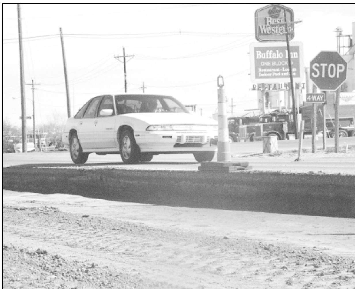
There is at least a one-foot drop off where the asphalt has been removed from K-27 at U.S. 24. Photo by Doug Stephens/The Goodland Daily News
