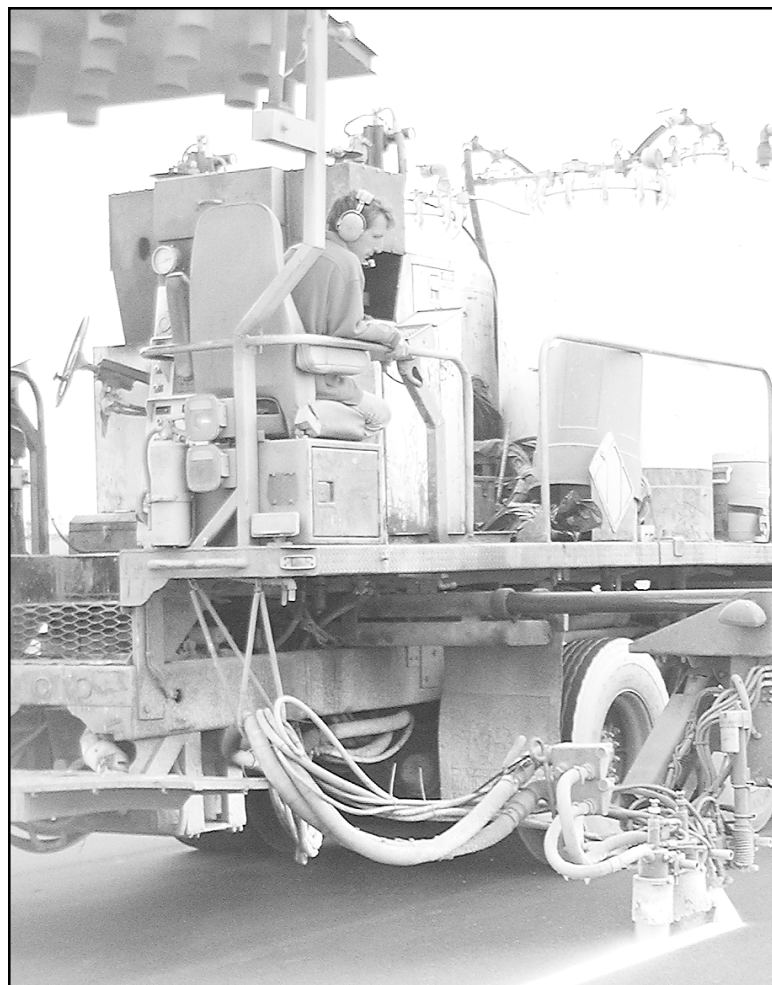
All Iowa, a company from Iowa, painted white and yellow stripes on the new section of K-27 north of Goodland this morning. Highway officials said the job should be finished today.
