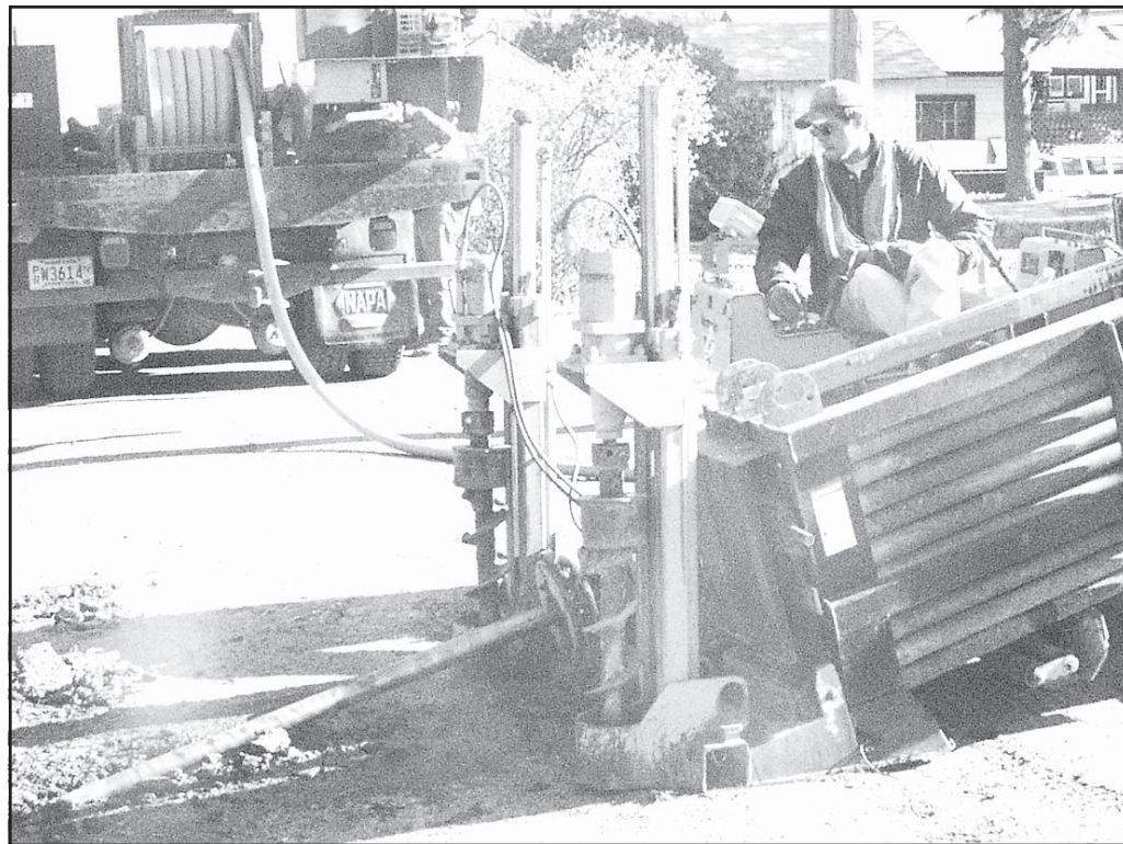
An S&T worker used equipment to drill holes near homes in Goodland to install cable. Photo by Doug Stephens/The Goodland Daily News
