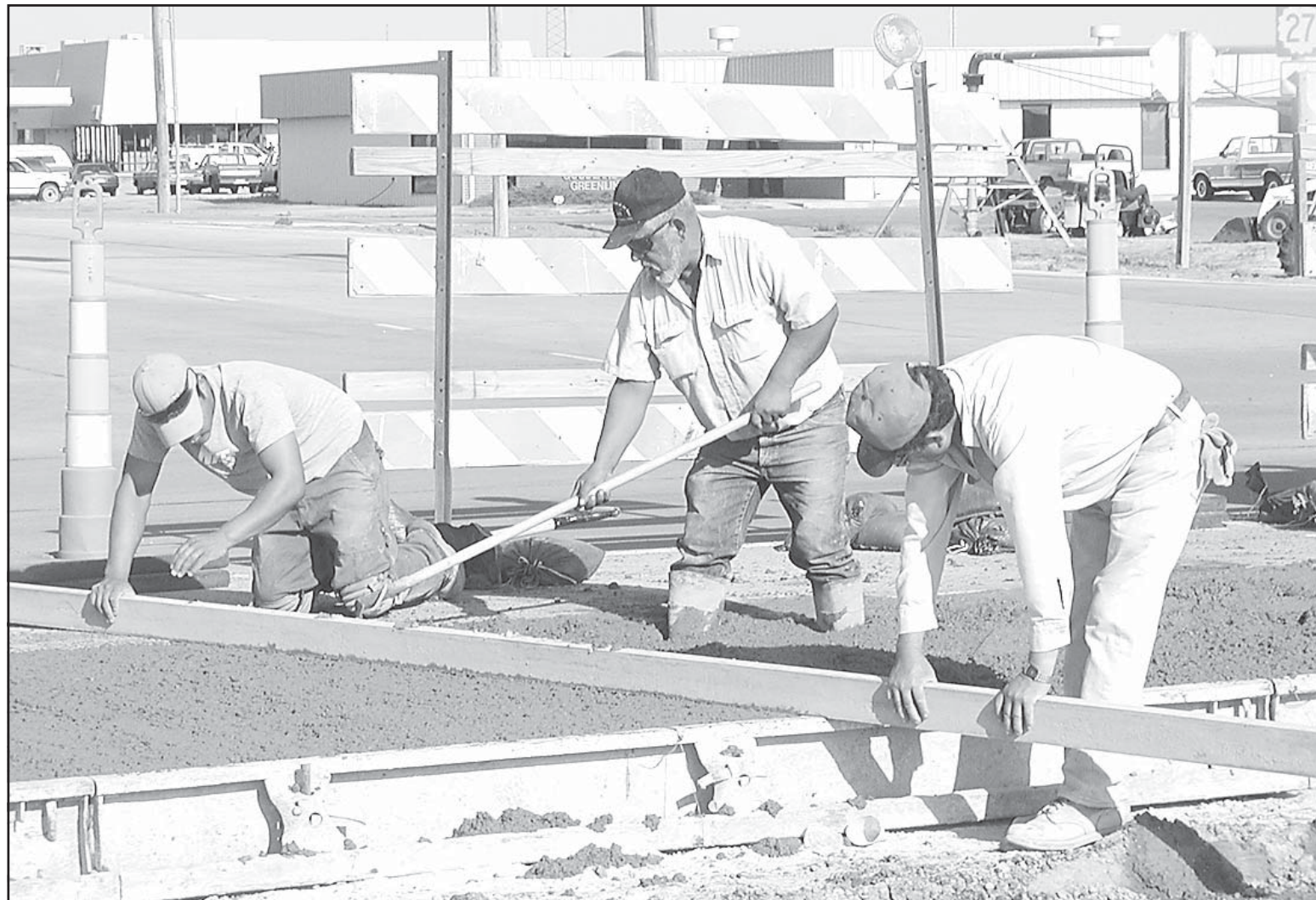
Workers from Ritchie Paving smoothed freshly poured concrete on K-27 last week. The whole U.S. 24/K-27 intersection should be repaved by Thursday, Aug. 1. Photo by Doug Stephens/The Goodland Daily News
