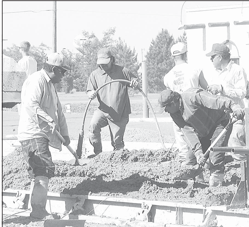
A worker with Cahoj Earthmoving of Atwood (left picture) tested the ground after the pavement was torn off of Cattletrail this spring. A crew from Ritchie Paving (above) shoveled wet concrete into place. Photos by Doug Stephens/The Goodland Daily News
