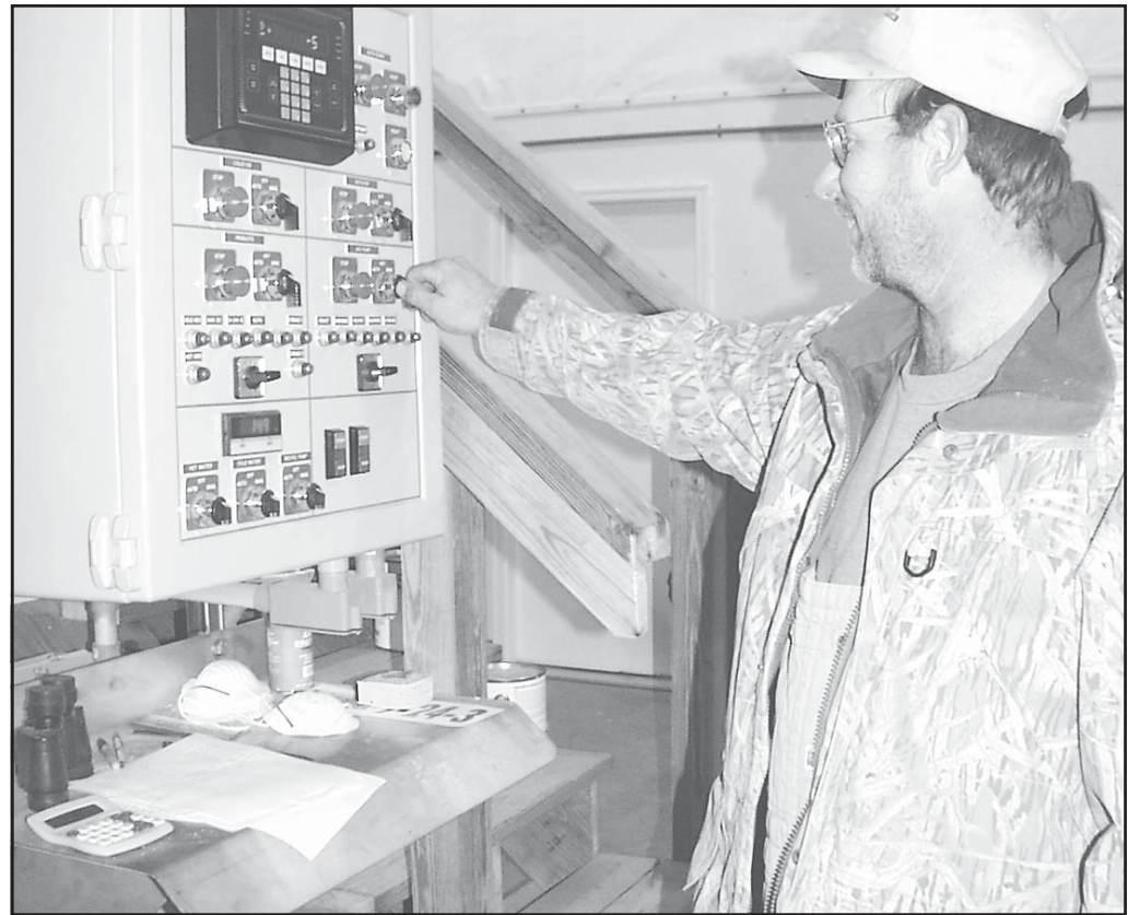
Danny Edwards, manufacturing supervisor, adjusted a panel which controls fertilizer ingredients at the Agro-Culture Liquid Fertilizer Plant.
