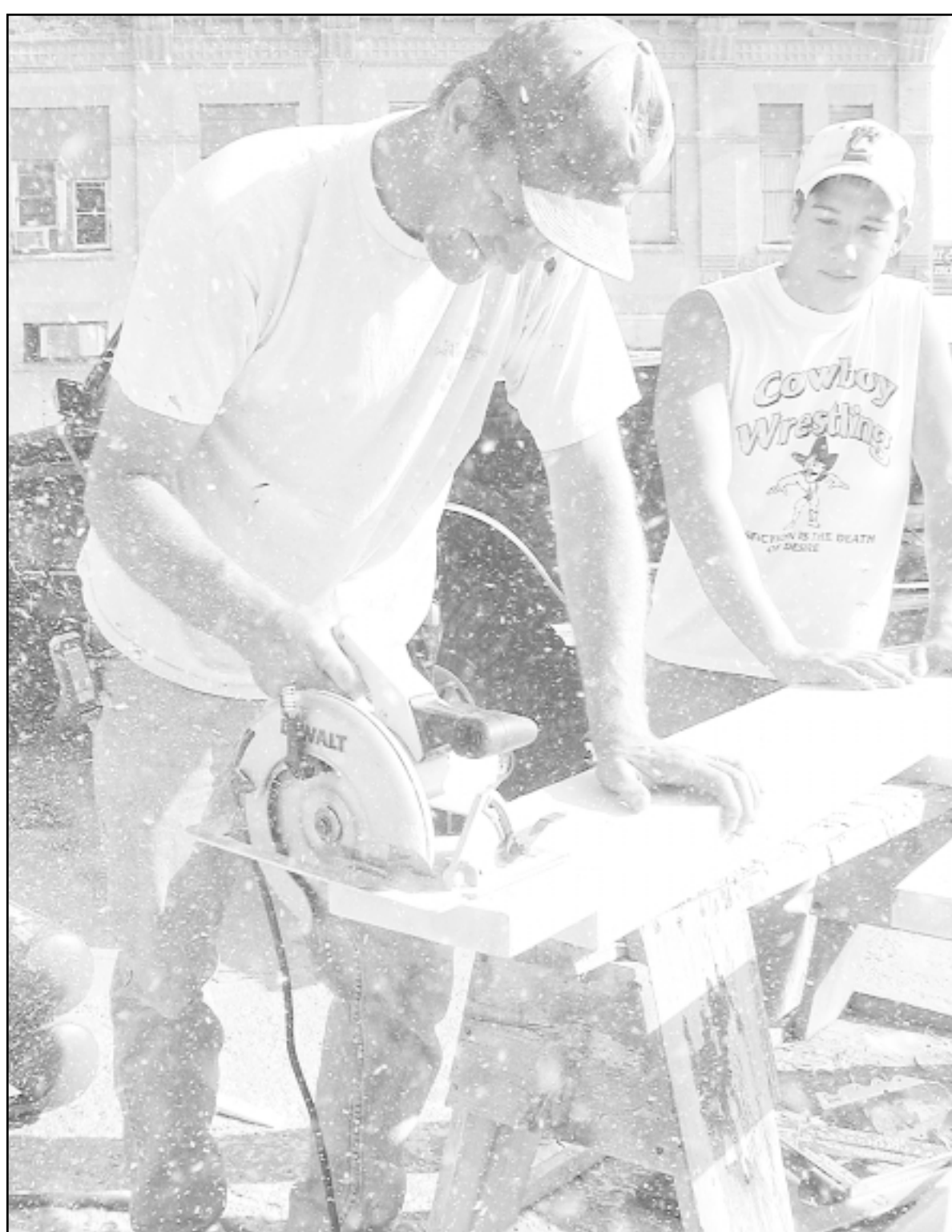
J.J. Howard, who works for WW Construction, used an electric hand saw to cut a board for the new awning on the old gas station building at 13th and Main, which is being turned into a Peoples State Bank. Malcolm White (in the background) was helping build the awning last week. The new bank is expected to open next month.
