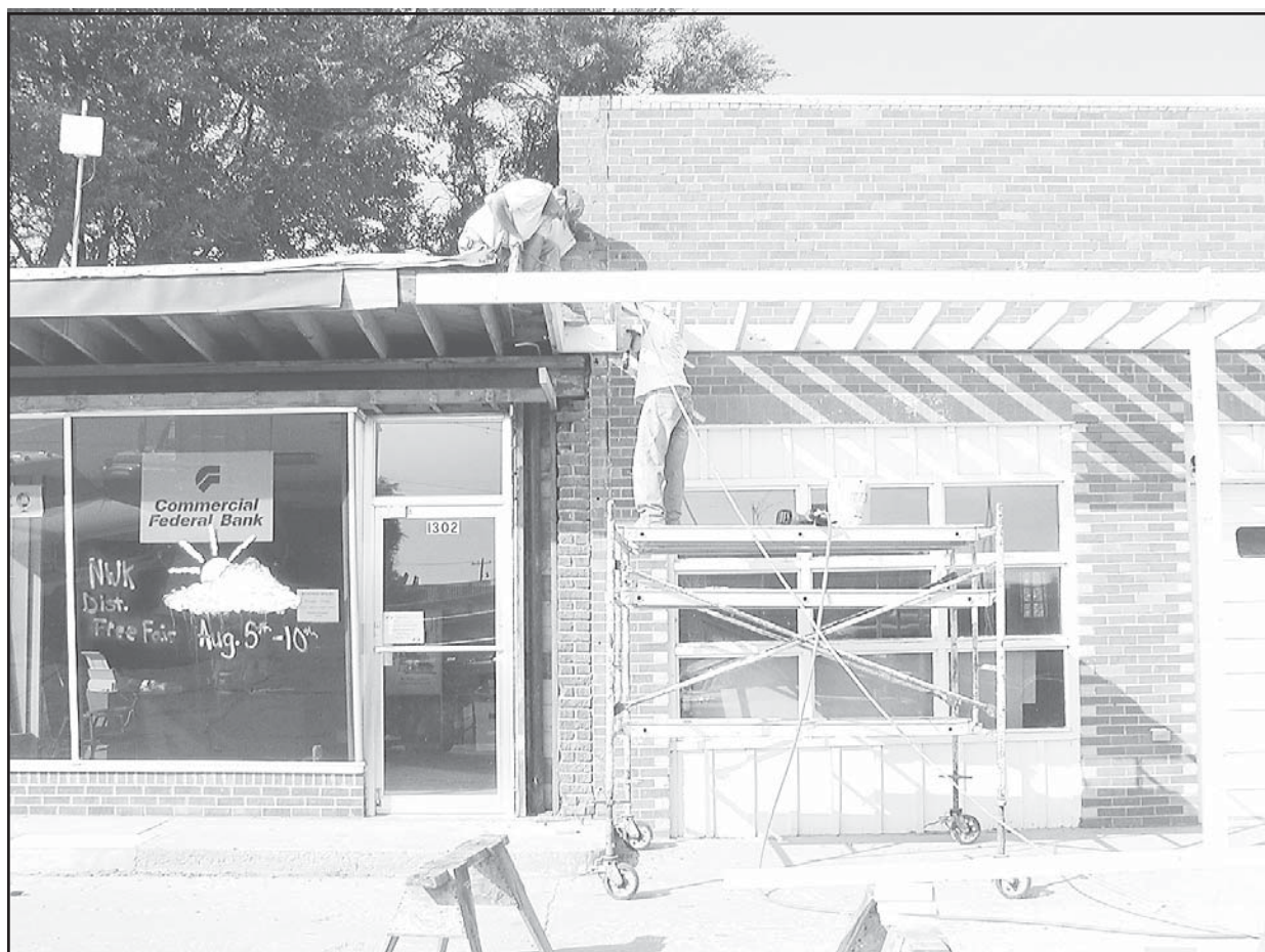
Workers with WW Construction built a new awning last week onto the building at 13th and Main that will soon be a Peoples State Bank. Photo by Rachel Miscall/The Goodland Daily News
